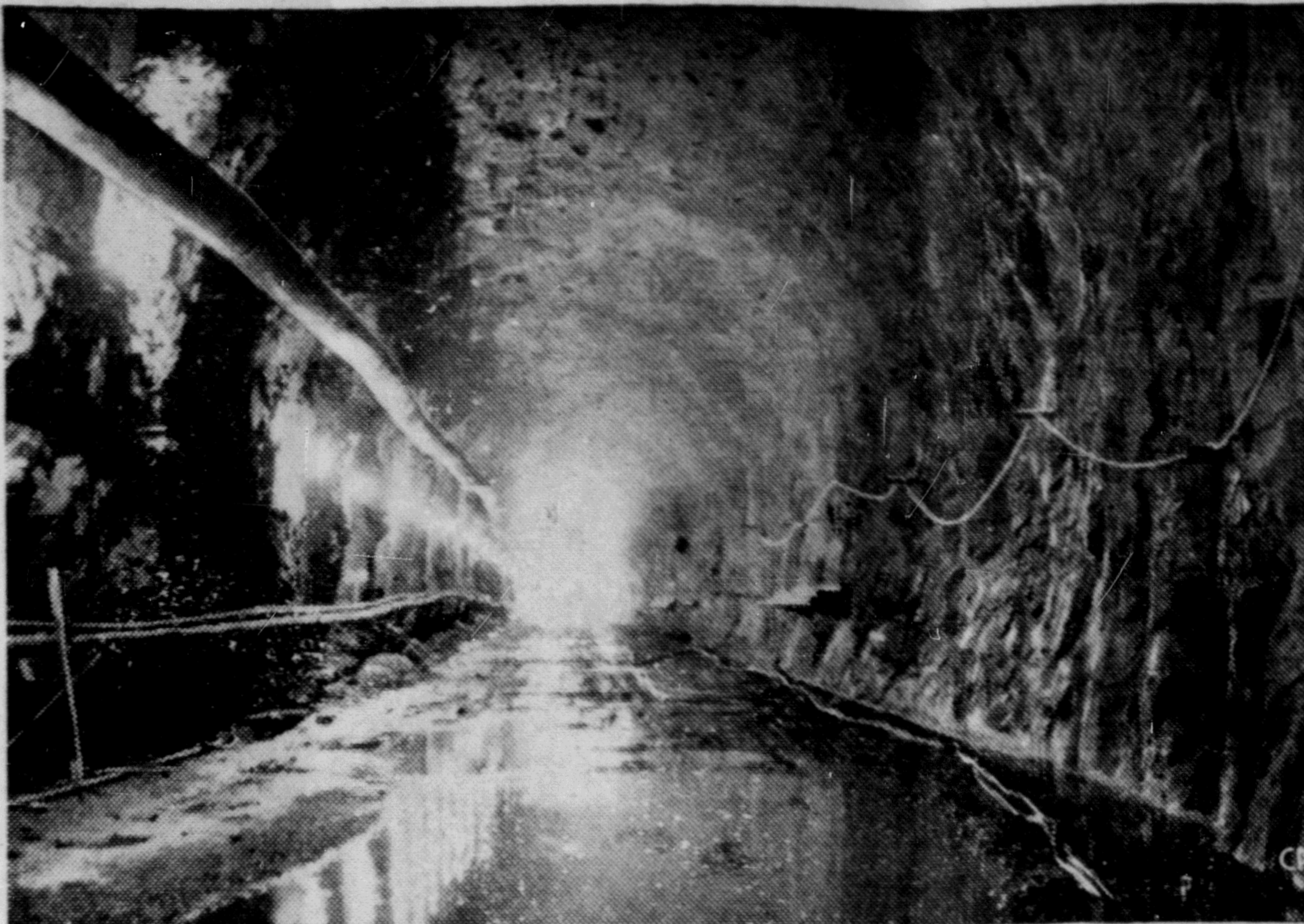
A TAIL-RACE TUNNEL, which channels water into the Kemano River, is one of a series built through the coast mountain range for the $550,000,000 aluminum industry under construction at Kitimat, B.C., 450 miles north of Vancouver. Water is backed up from the Nechako dam to create a 350-square-mile watershed and is carried through a tunnel to the power site 125 miles west of the dam. The water then is carried off through a tail-race tunnel to the Kemano River which joins the Pacific Ocean at Gardner Canal. (CP PHOTO)
