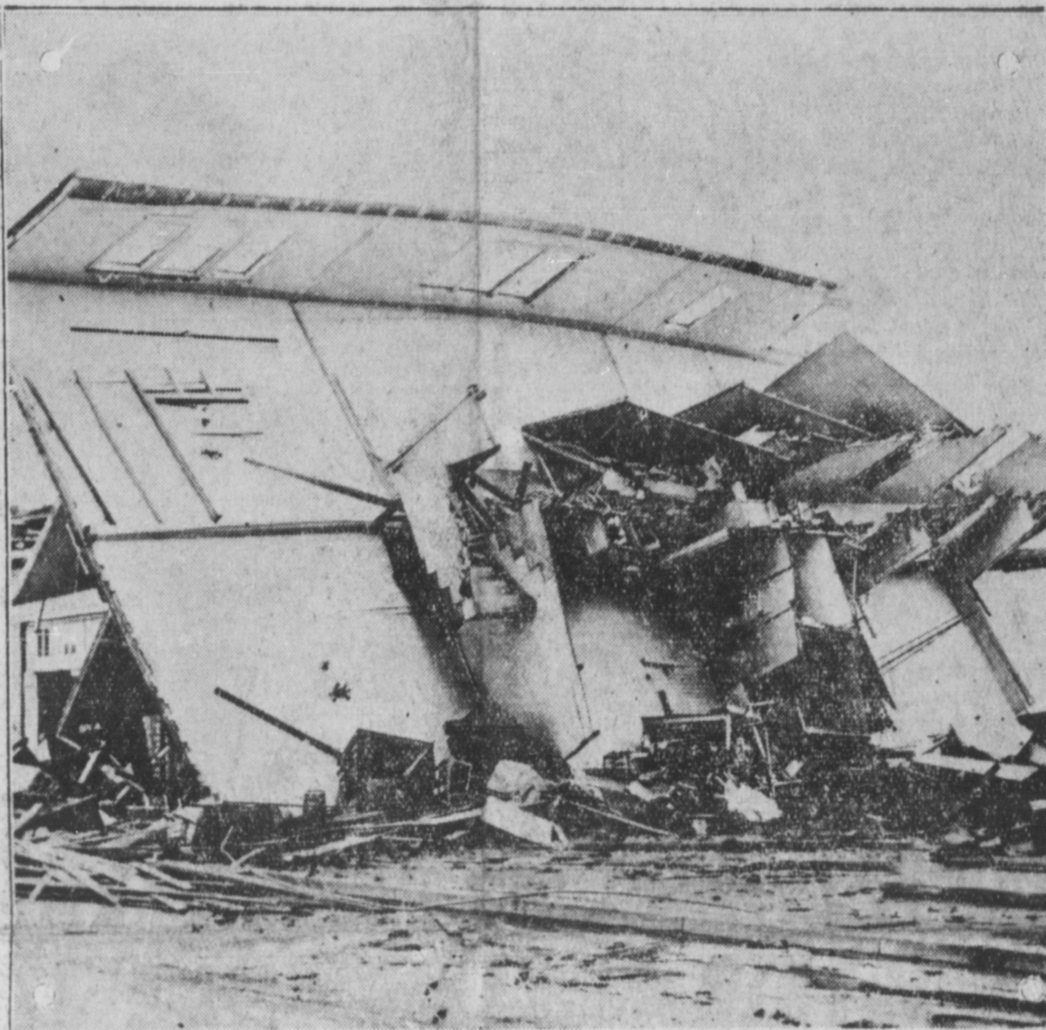
When a Texas hurricane comes to town, the natives generally know about it. Here is all the wind left of what was once a stout two-storey structure. Seventeen people were killed in the recent big blow.
