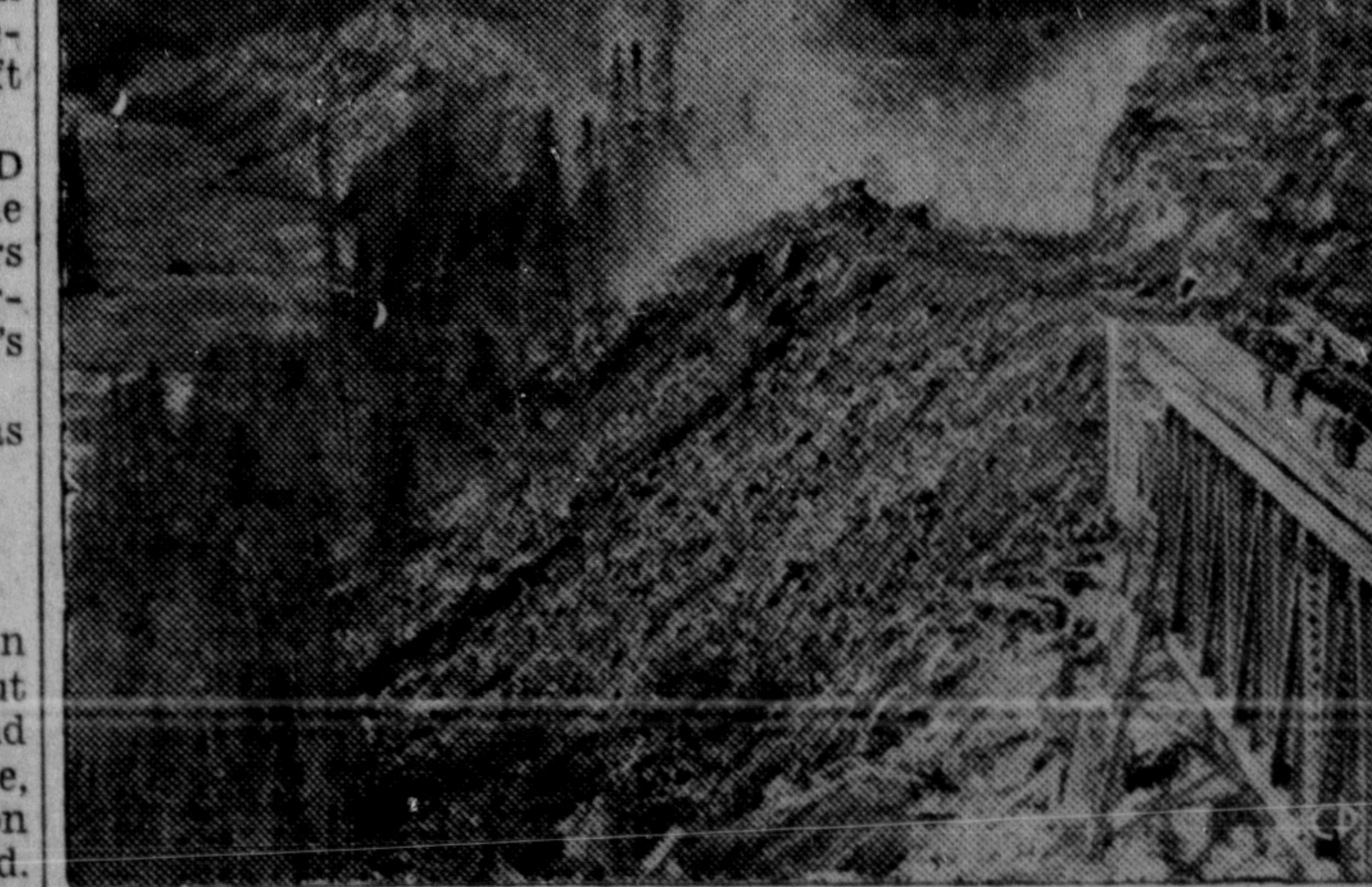
BRIDGE MOISIE—The Moisie River, another of the grim barriers encountered in the battle to develop the Labrador-Ungava iron, finally has been spanned. (CP PHOTO)
