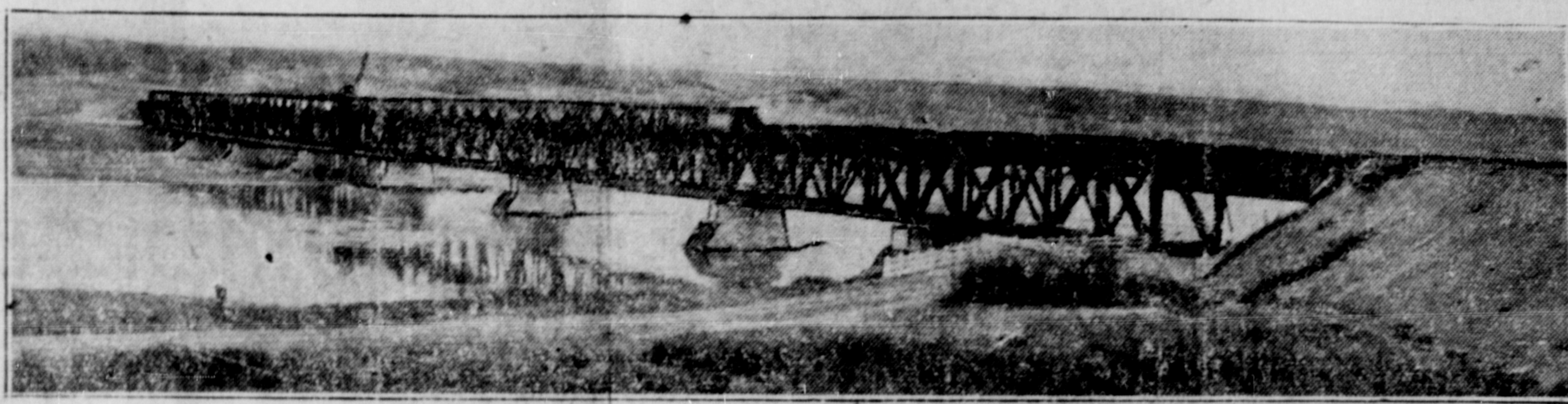
This bridge at Dunblane in Saskatchewan will complete the branch line of the Canadian National Railways linking Central Butte on the Riverhurst sub-division with Dunblane on the Conquest sub-division. The bridge is to be opened this month and Boards of Trade of Regina, Moose Jaw and Saskatoon will participate in the opening. The bridge, which has been under construction for two years and which will carry vehicular as well as rail traffic, and branch line will effect very considerable mileage saving and will provide for a more direct routing of coal and other materials over the lines of the Canadian National to and from points in southwestern Saskatchewan and southern Alberta. There are ten spans supported by nine concrete piers and two abutments.
