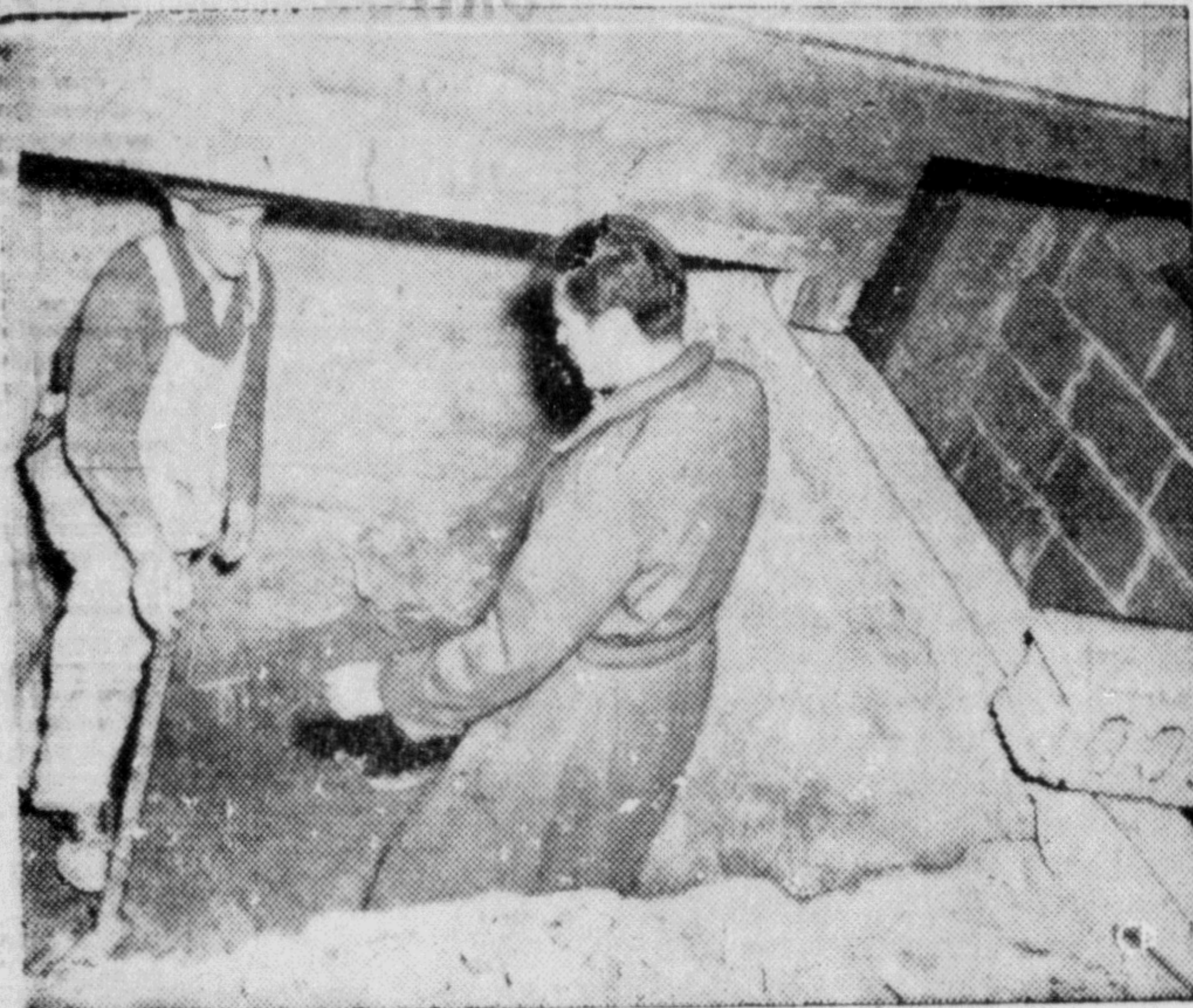
CAUTIOUS RESIDENT —This excavation under the garage of a new house in Lethbridge, Alta., is designed as an atom-bomb shelter. When completed, it will have three-foot concrete walls and its own air-conditioning system. Seventeen-year-old Norman Wiebe, left, explains the layout of the shelter to a reporter. (CP PHOTO)
