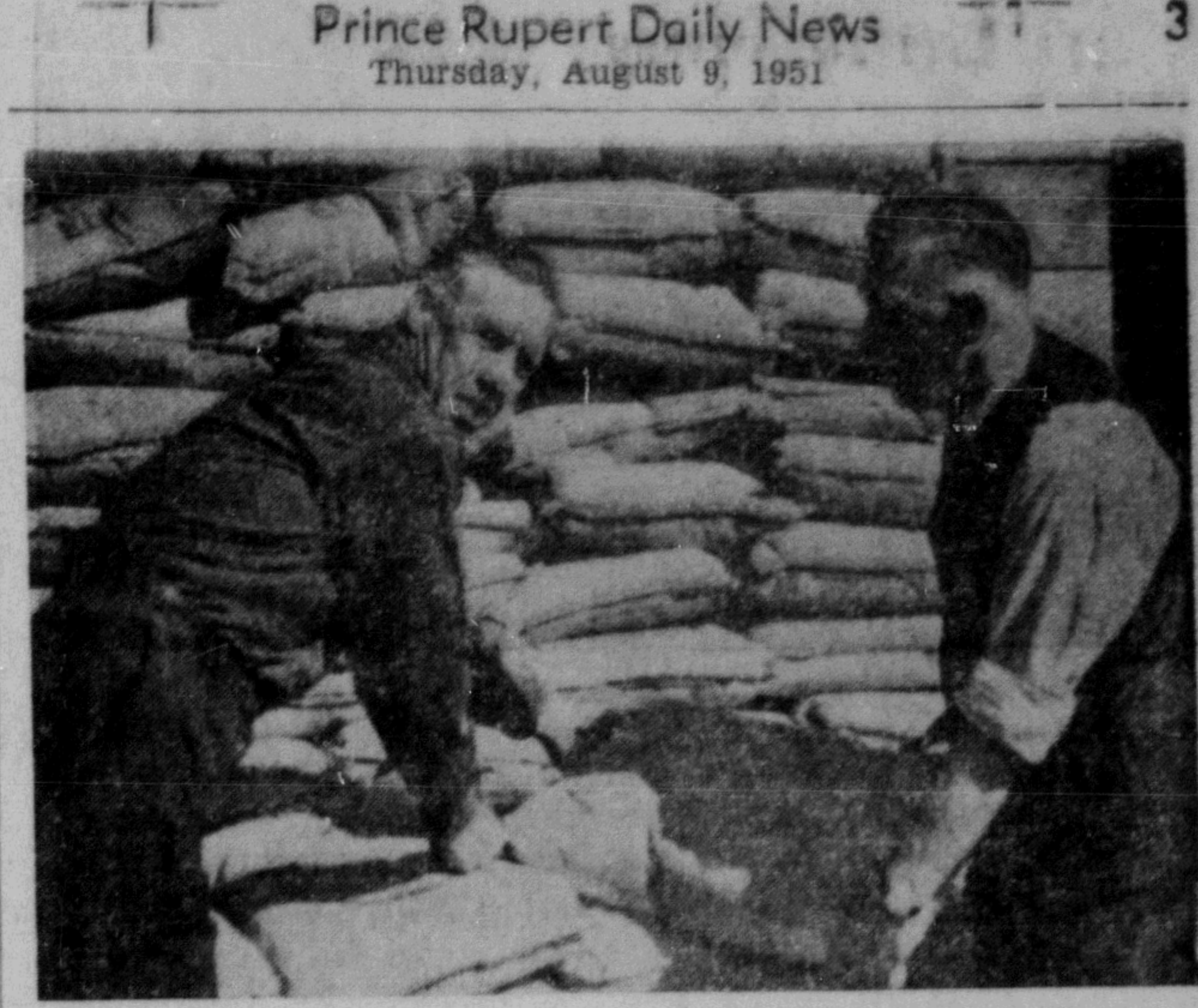
FIRST HOME OF 20 to be built by Celco Co-operative Housing Association, Port Edward, is getting its concrete foundation laid and further work is well under way. Here President Len Loucks and Secretary-Treasurer Fred Gray are handing bags of cement to the mixer. Mr. Loucks is electrical superintendent for Columbia Cellulose Co. Ltd.; Mr. Gray, an engineer.
