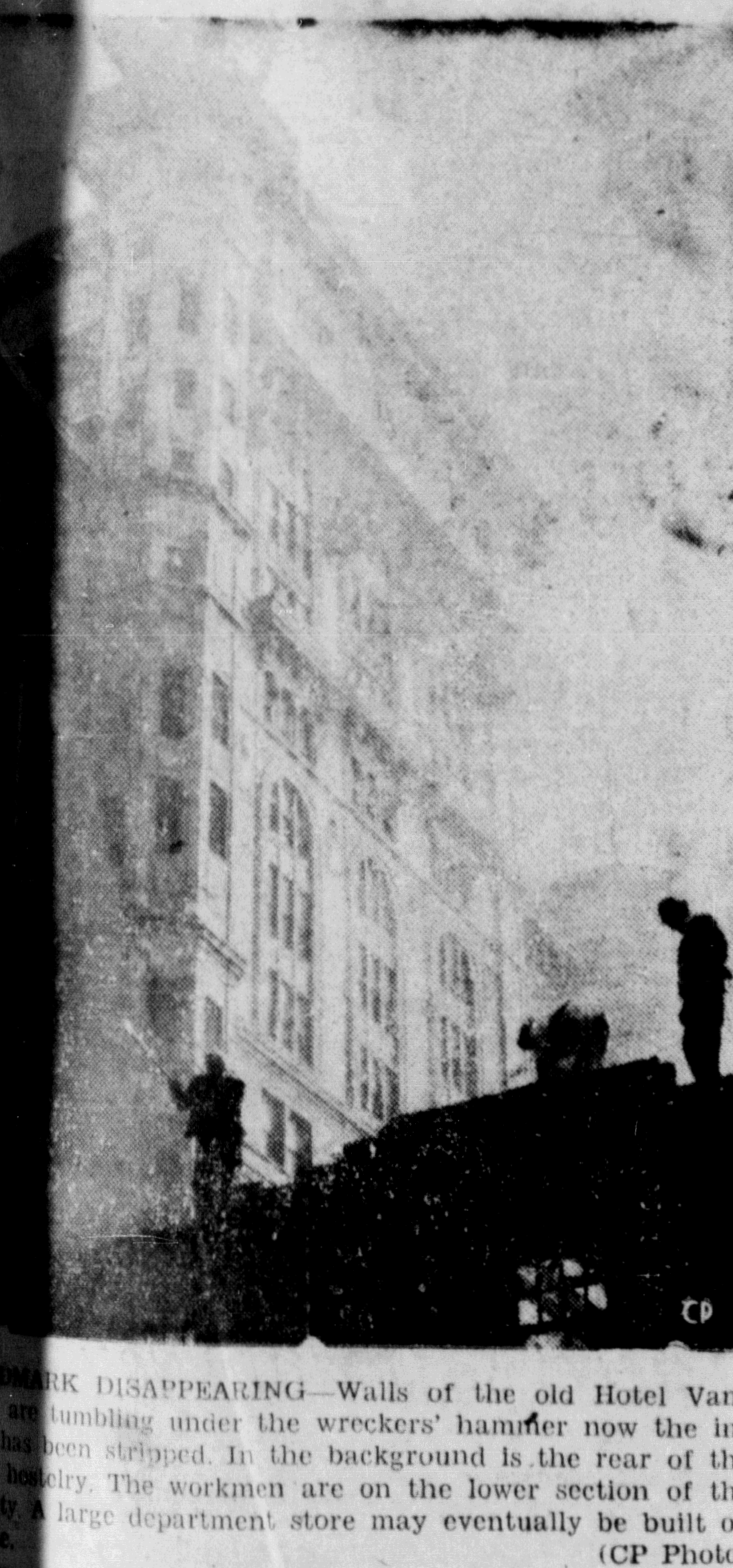
MARK DISAPPEARING—Walls of the old Hotel Vancouver are tumbling under the wreckers' hammer now the building has been stripped. In the background is the rear of the new building. The workmen are on the lower section of the building. A large department store may eventually be built on the site. (CP Photo)
