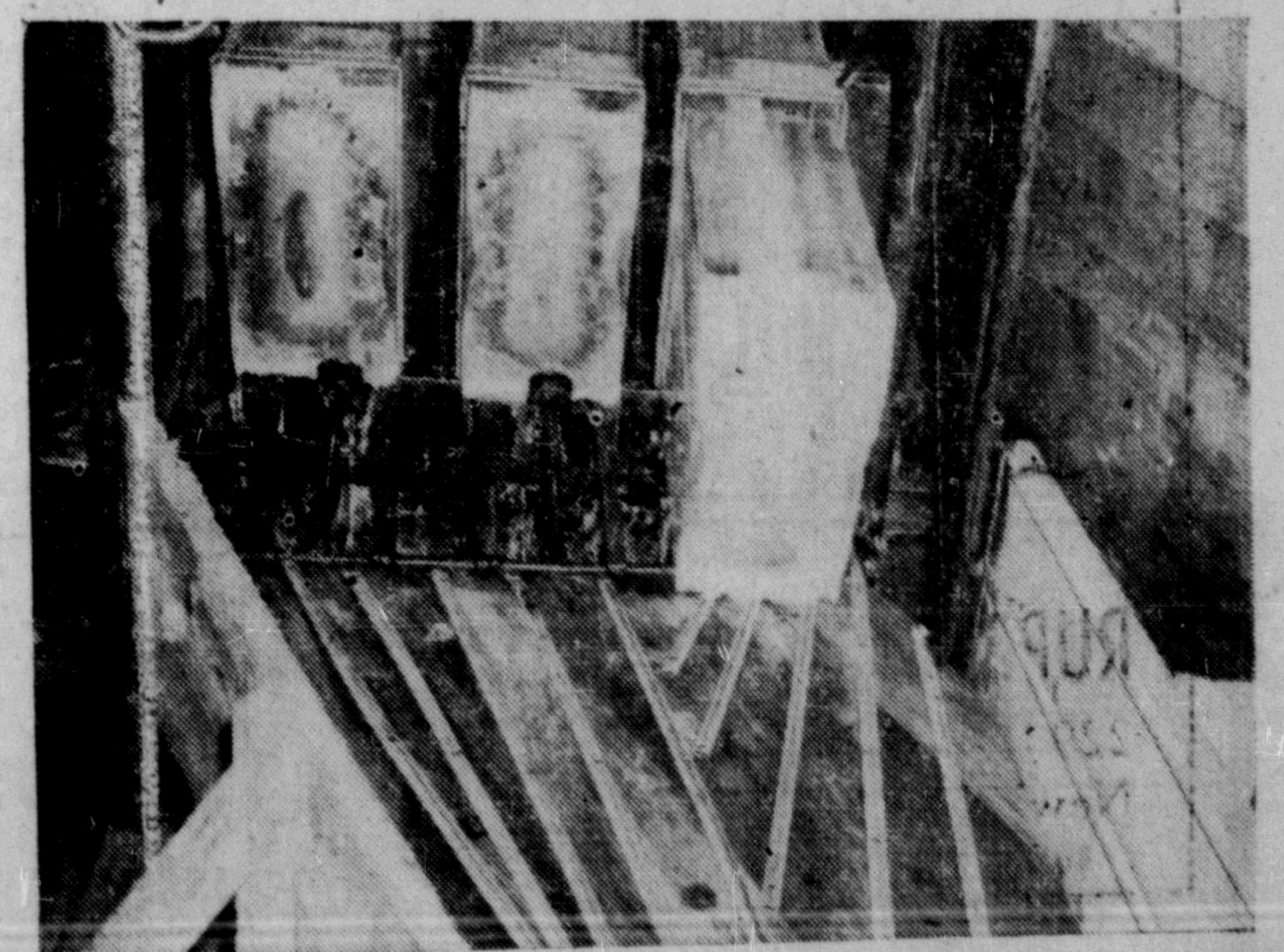
THE ICE PLANT—Makes over 30 tons per day
