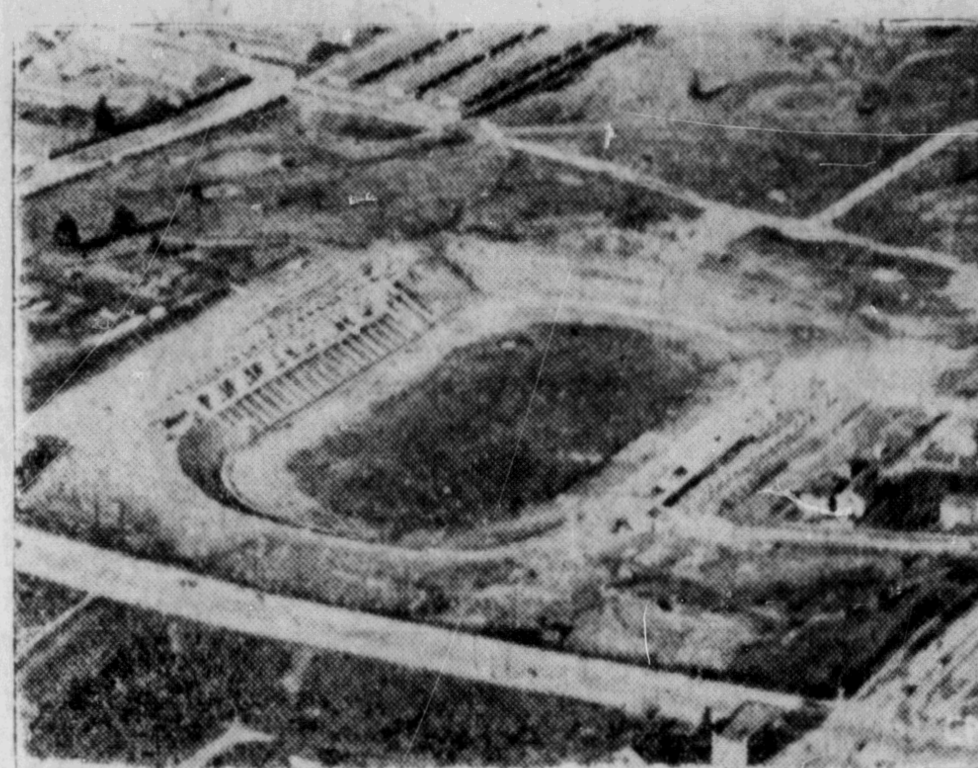
THIS AERIAL VIEW shows construction progress on Canada's largest stadium, to be used for the British Empire Games at Vancouver next summer. To cost $1,895,000 and scheduled for completion April 30, three months before the games start, it will hold 35,000 with 10,000 seats under cover.
