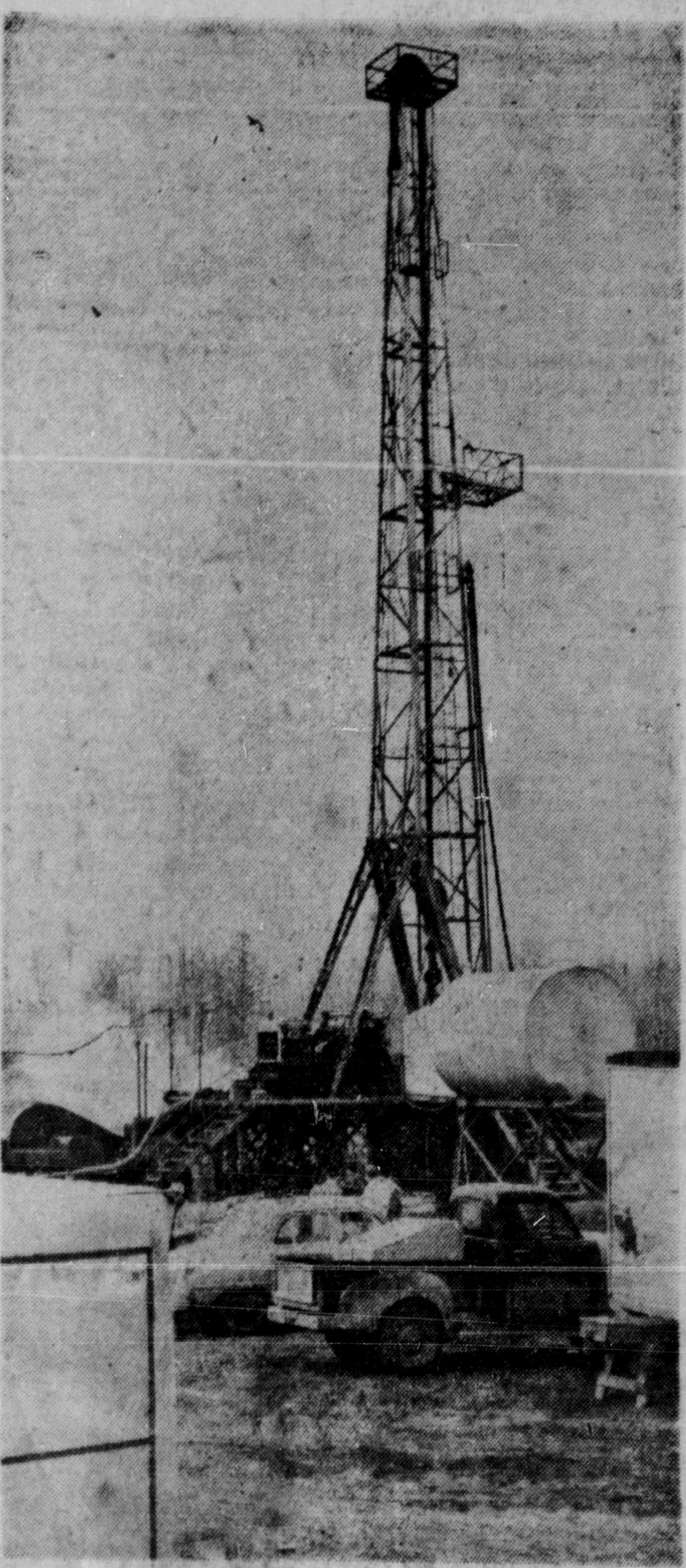
THE OIL FEVER which has gripped B.C.'s neighboring province of Alberta since the end of the war has spread into B.C. borders. Exploration and drilling is increasing. Above, is the drilling operation at the Pacific Fort St. John No. 6 well in northeastern British Columbia.
