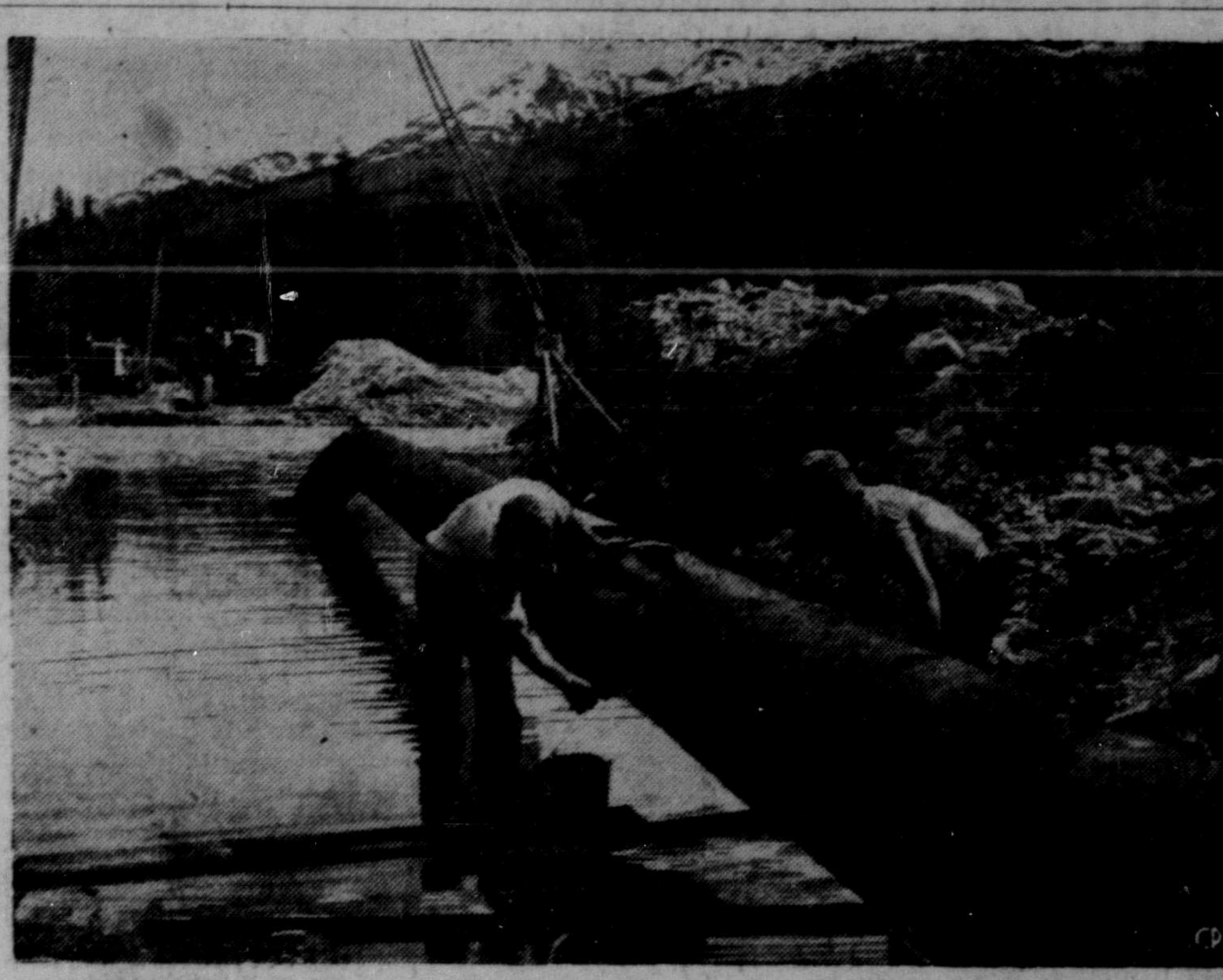
OIL PIPELINE —A pipeline is being laid from Edmonton to Vancouver, 711 miles, to find new markets for western oil. This picture shows a crossing of the upper Fraser river in the Rocky Mountains. It is one of 60 river crossings along the line, owned by the Trans-Mountain Oil Pipeline Company. (CP PHOTO)
