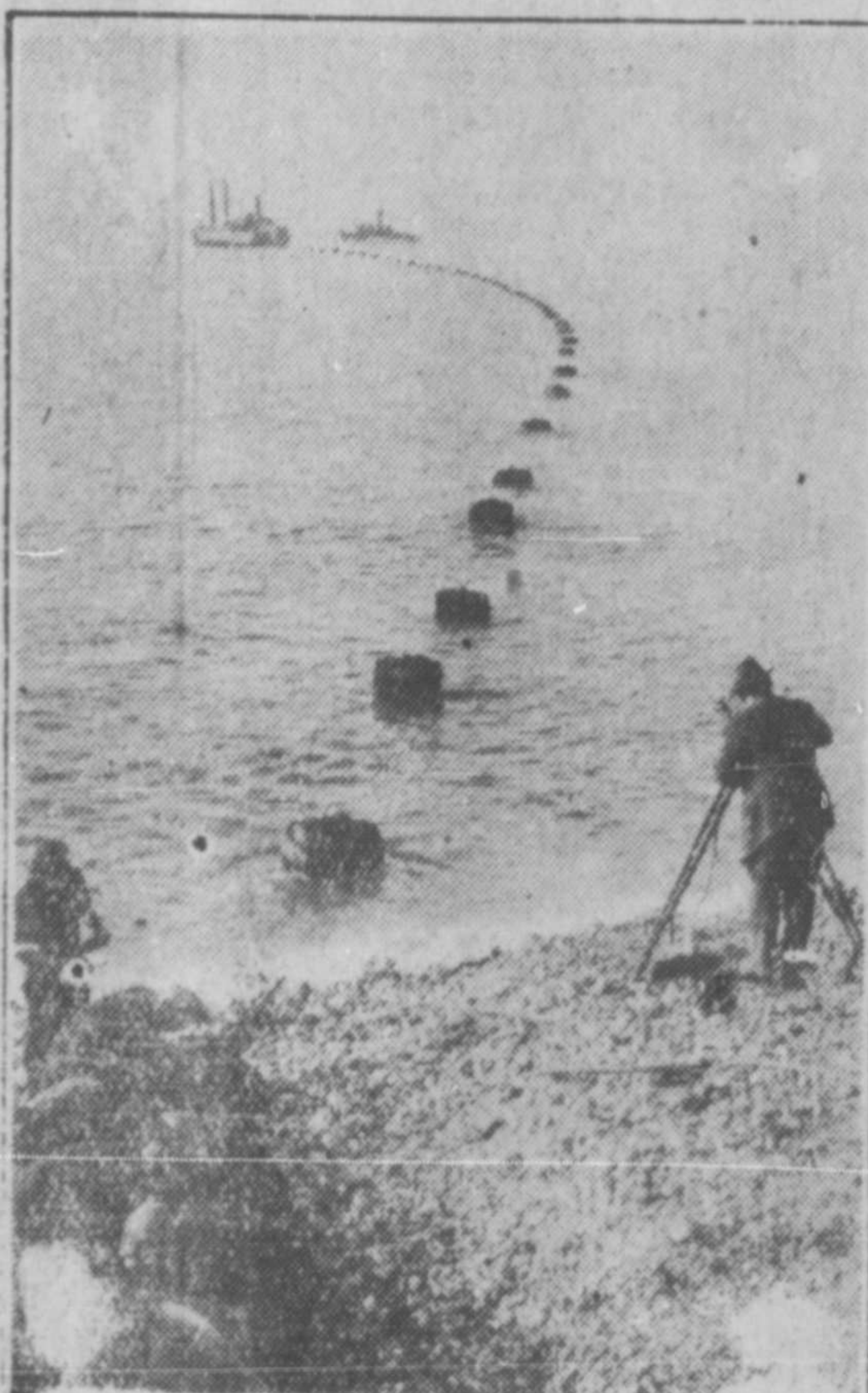
LAYING THE LAST LINK of direct cable from France to America. The S.S. Colonia connecting La Havre, France and Penzance, England, where the present cable ends
