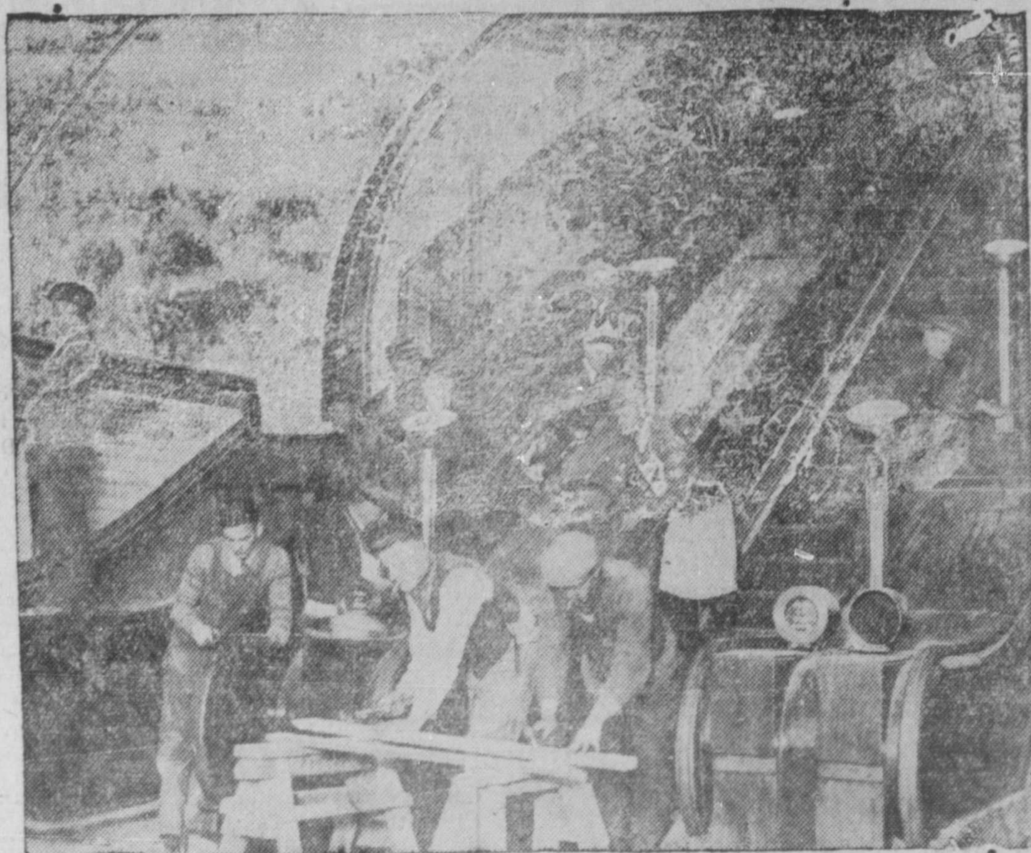
The above picture shows workmen putting the finishing touches to some of the escalators of the Piccadilly Circus New Underground Station, London, which has taken four years to build. This new station, cost more than $2,000,000 to construct.
