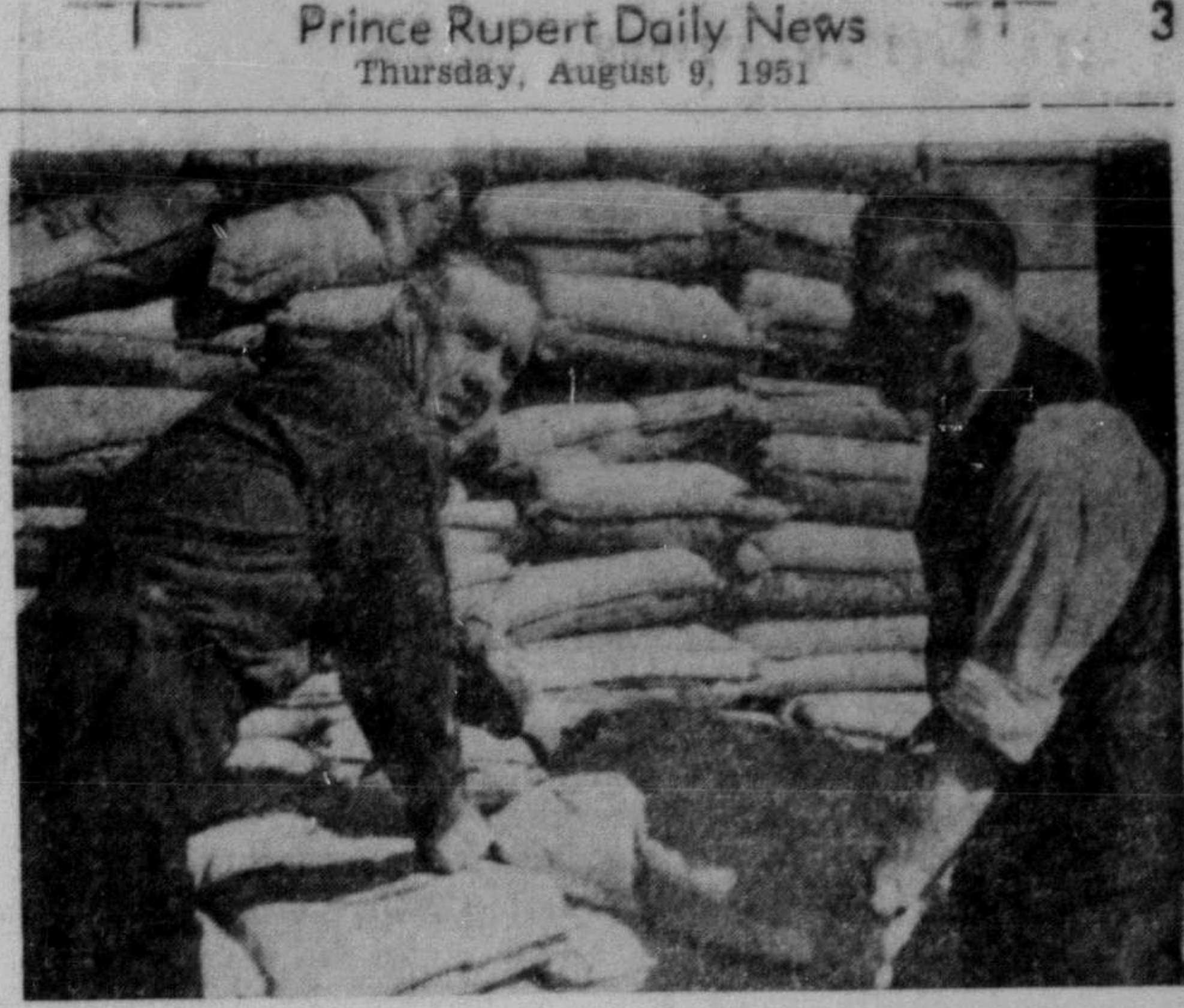
FIRST HOME OF 20 to be built by Celco Co-operative Housing Association, Port Edward, is getting its concrete foundation laid and further work is well under way. Here President Len Loucks and Secretary-Treasurer Fred Gray are handling bags of cement to the mixer. Mr. Loucks is electrical superintendent for Columbia Cellulose Co. Ltd.; Mr. Gray, an engineer.
