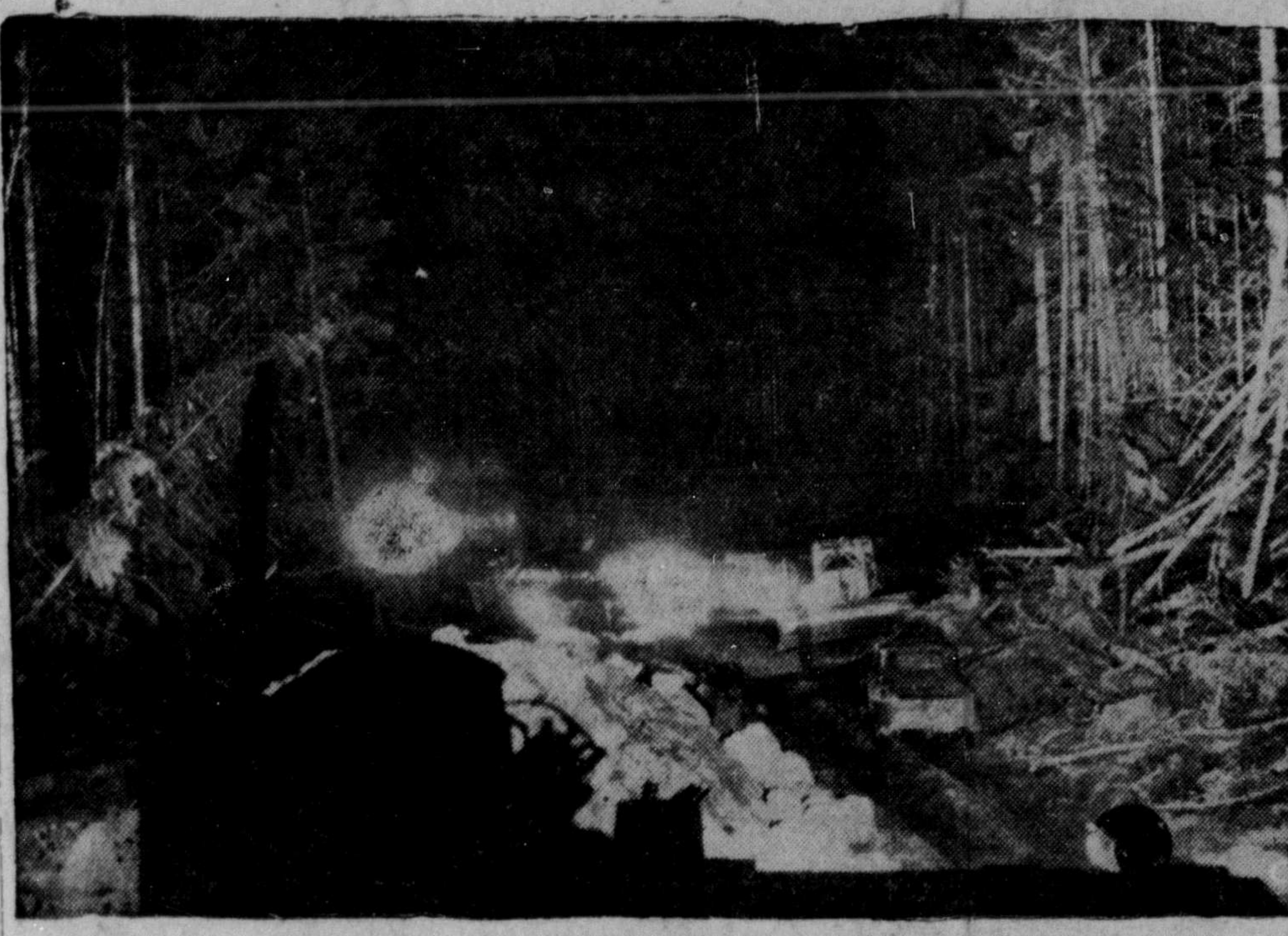
NIGHT WORK—Work continues under floodlights on the Kemano Road in Gardner Canal, first step in development of a section of northern British Columbia for an aluminum plant, first phase of which will cost $160,000,000. The 11-mile road heads through practically-unknown mountain country. (CP PHOTO)
