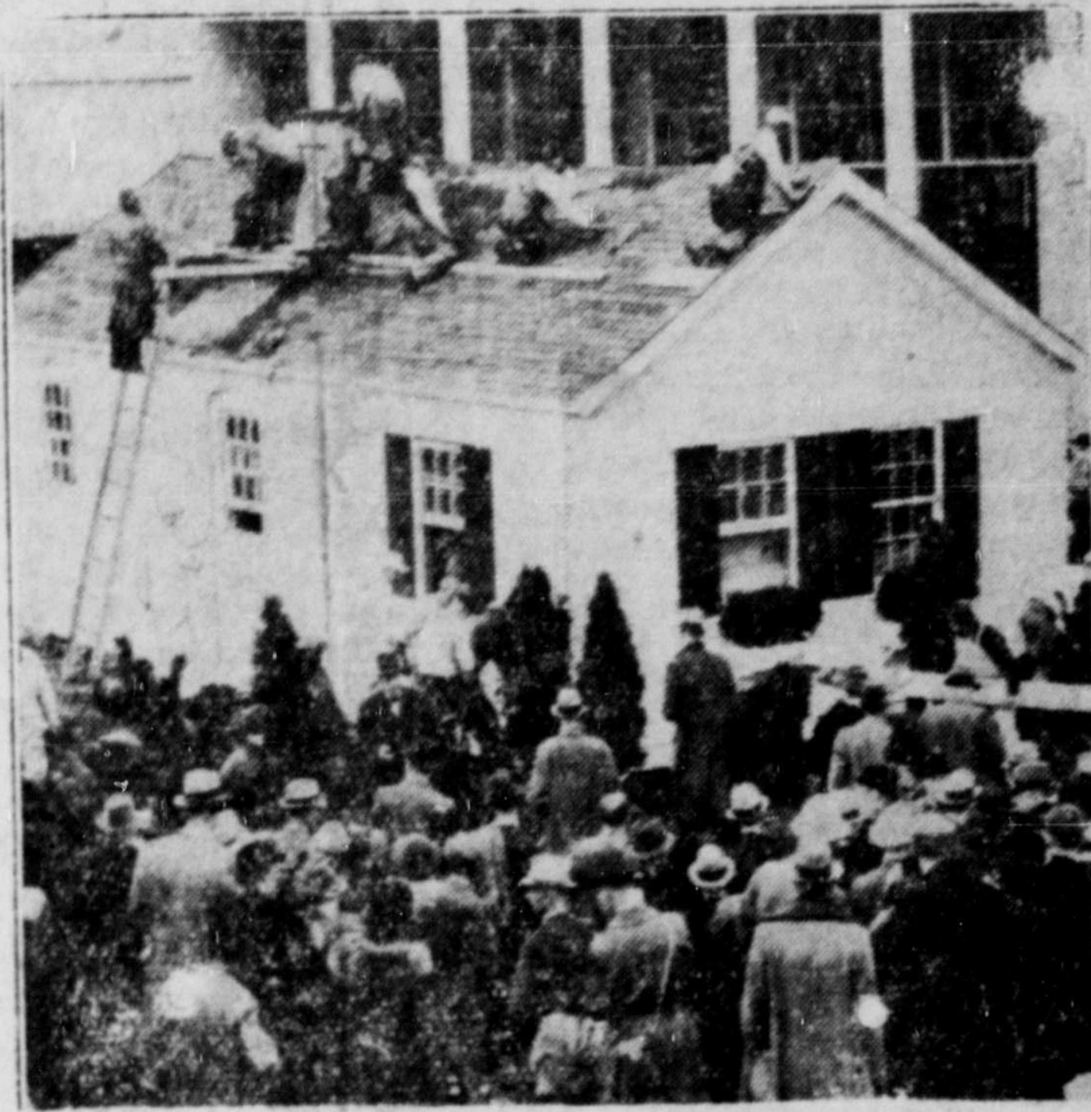
Roofers are putting the finishing touches on this modernized Cape Cod cottage in Chicago, which they built in the record time of seven hours as thousands viewed their efforts.
