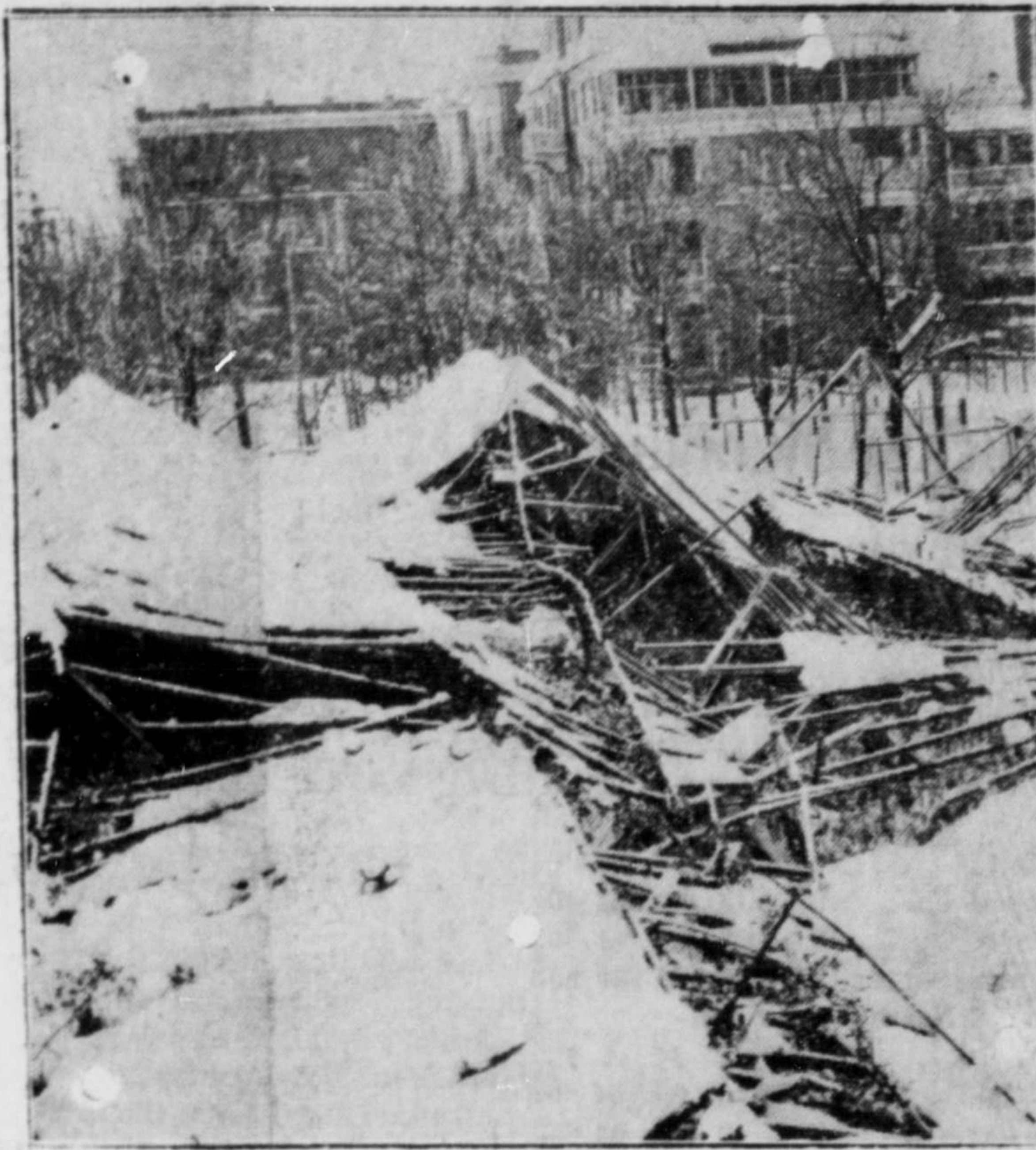
Twenty-five thousand panes of glass crashed down when six greenhouses collapsed under the weight of an eight-inch snow which fell in as many hours in Edmonton, adding greatly to the already near-record depth. The heavy blanket, falling when it did, just at the end of a month of real sub zero weather when the mercury slipped to 44 below, greatly hampered the work of crews repairing frozen sewer and watermains.
