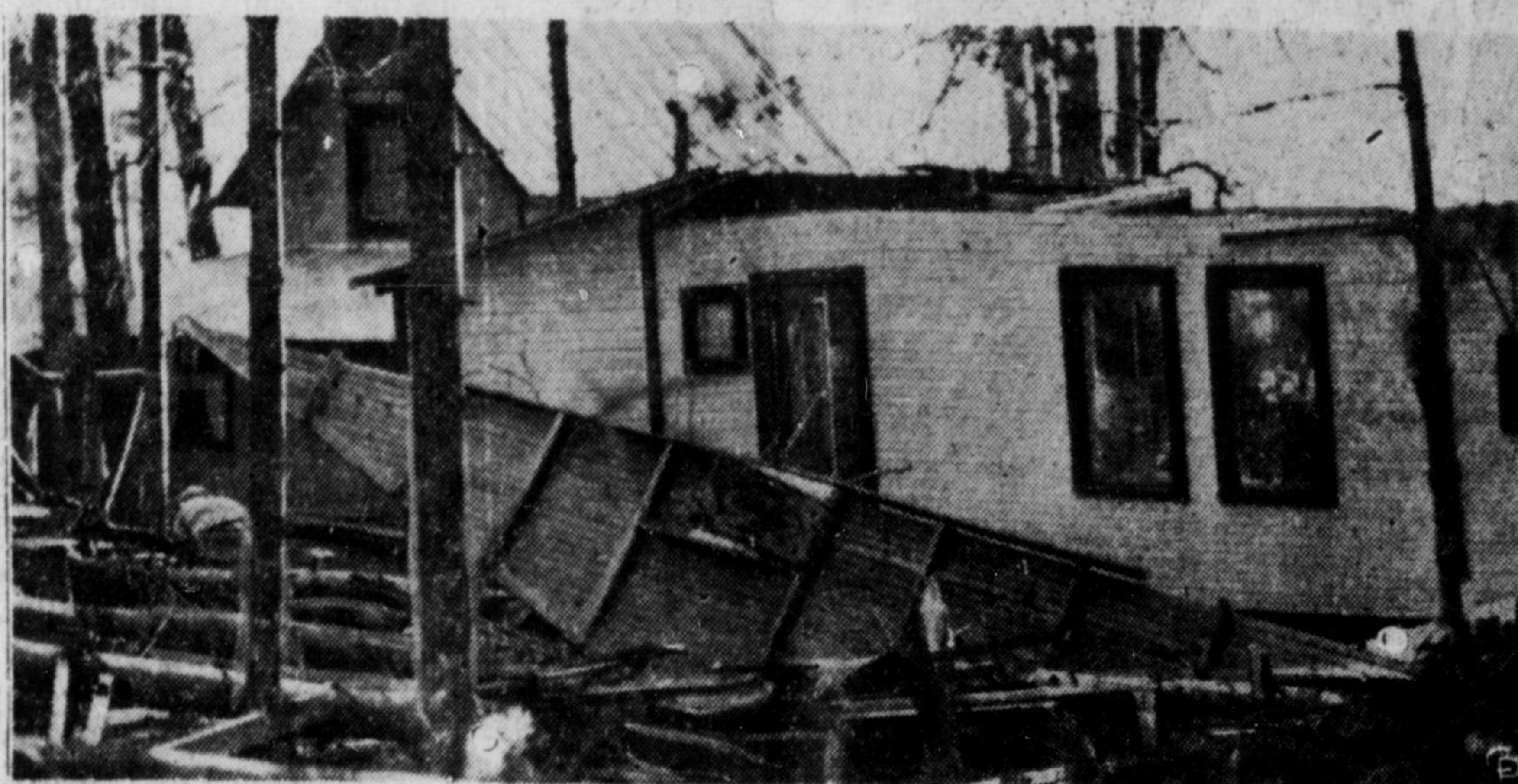
Only the fact that the summer resort at Norway Bay, near Ottawa, was depopulated saved many lives as tornado struck the colony, doing much damage. Above is shown cottage with roof blown off. The cottage was occupied, but none was injured.
