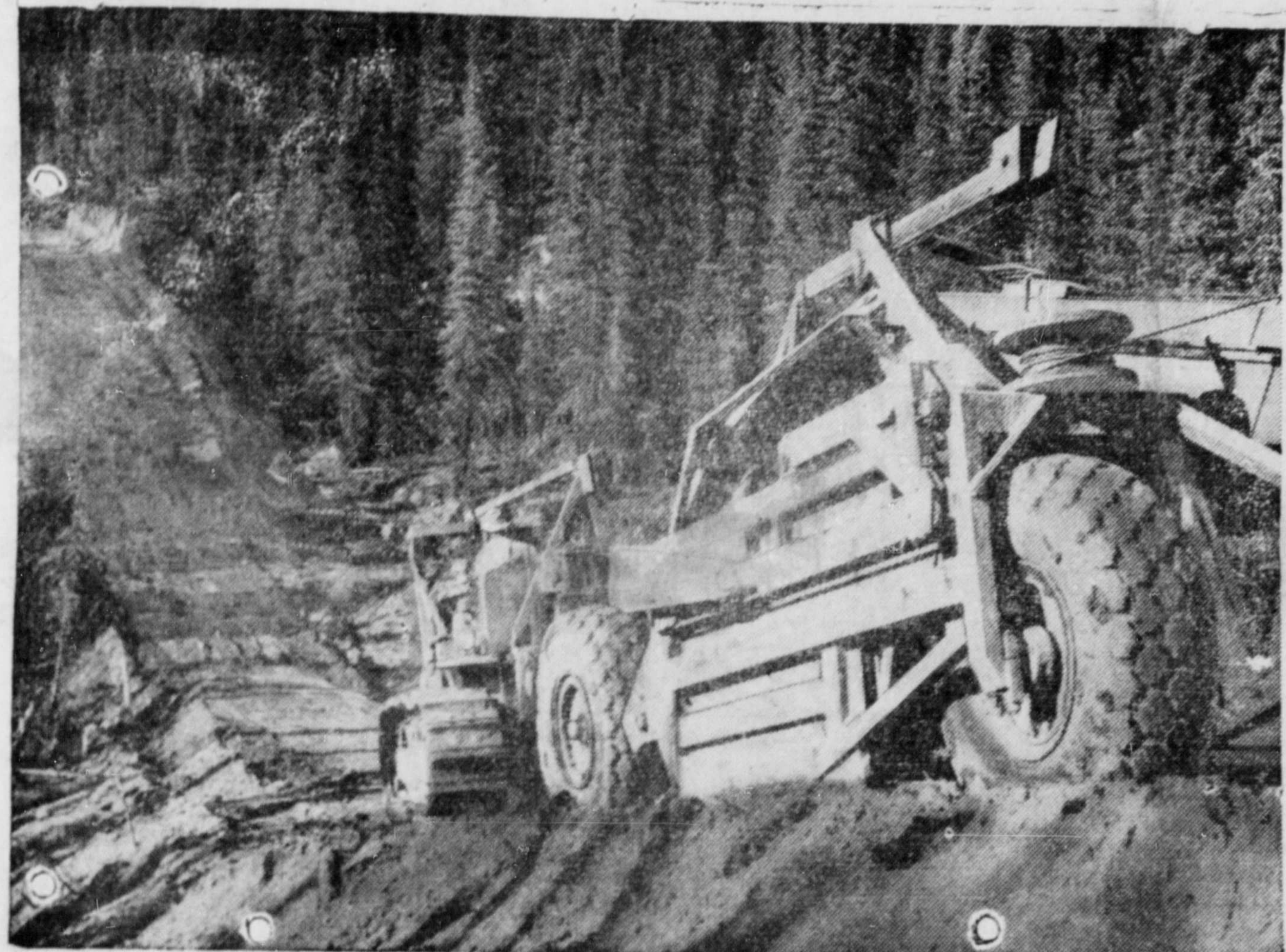
On this "carry-all" tons of earth are moved from one section of the road to a fill. Hidden two or three feet under the muskeg in some sections along the road are glacial ice formations thousands of years old. When muskeg is removed the ice melts, creating heavy morass. U.S. Army engineers have solved the problem. Bishop G. A. Rix tells of work on the Alaska in an interview published today.
