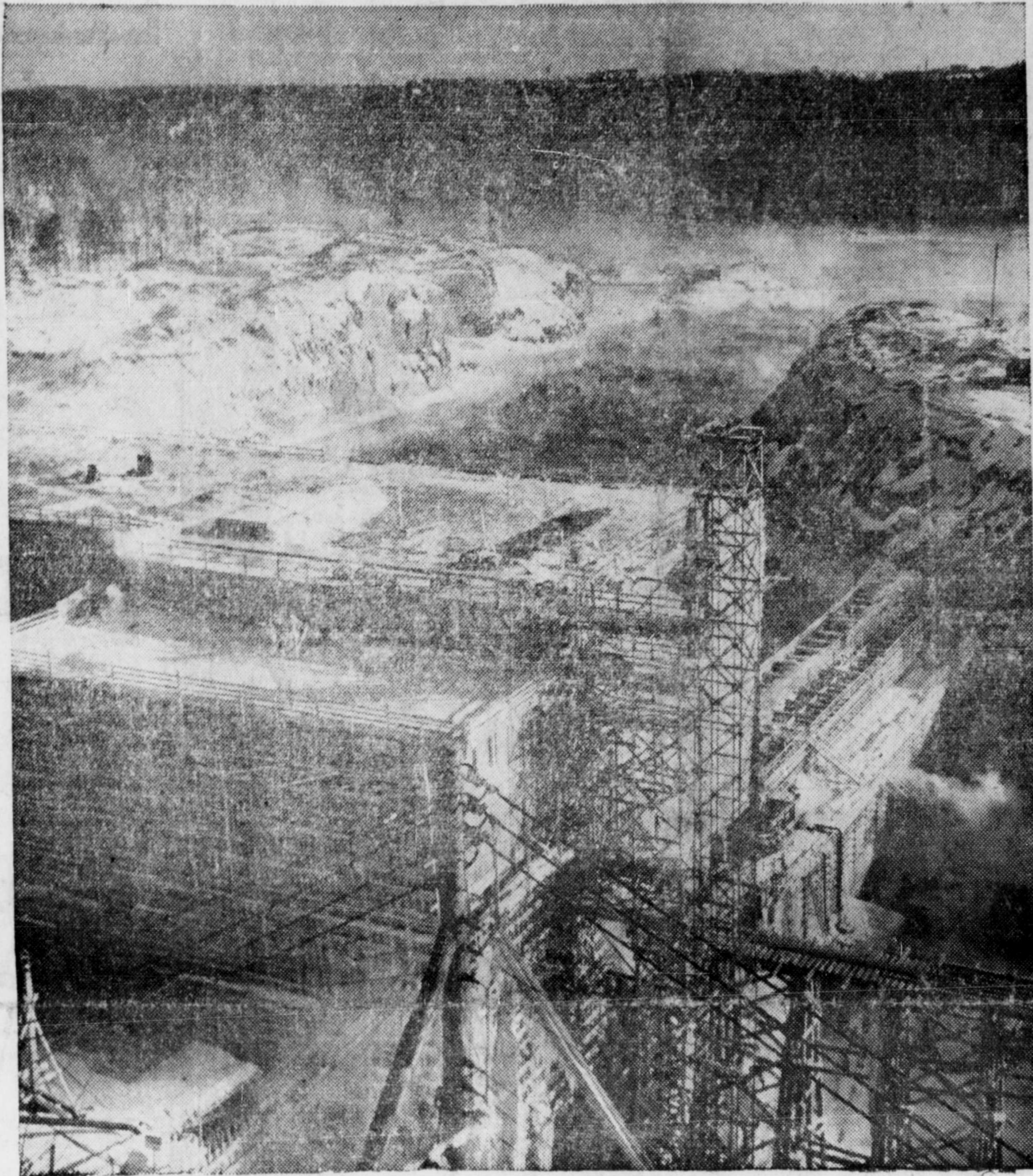
The dynamite used for blasting this huge rock cut would provide enough block-busters to blow Berlin to bits. This view shows tail race leading into the first half of powerhouse of the new Saguenay power project in Quebec. It will develop power while second being built. Cold mist rising from water is result of 50-below temperature when picture taken.
