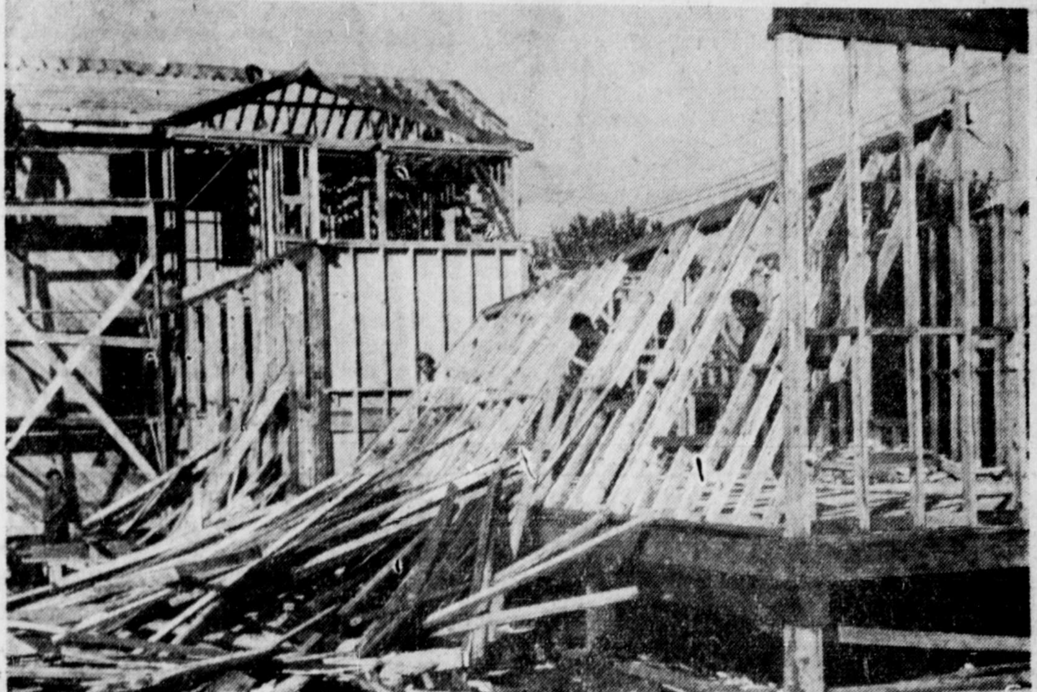
NOBEL, ONT., WAR PLANT SUPPLIES LUMBER FOR VETS' HOMES —A large section of wall framing, comprised mostly of valuable two-by-fours, comes crashing down as workmen take apart an 88-room women's staff house in Nobel village, Ont., in the course of recovering valuable building materials for veterans' housing in many parts of the province. At Nobel, a short distance north of Parry Sound, more than 226 buildings, formerly used in the manufacture of high explosives for Canada's share in the war, are being dismantled. All materials suitable for house building are being channelled into government-approved low-cost housing projects for veterans by the Central Mortgage and Housing Corporation. War Assets Corporation is handling the demolition and sales.
