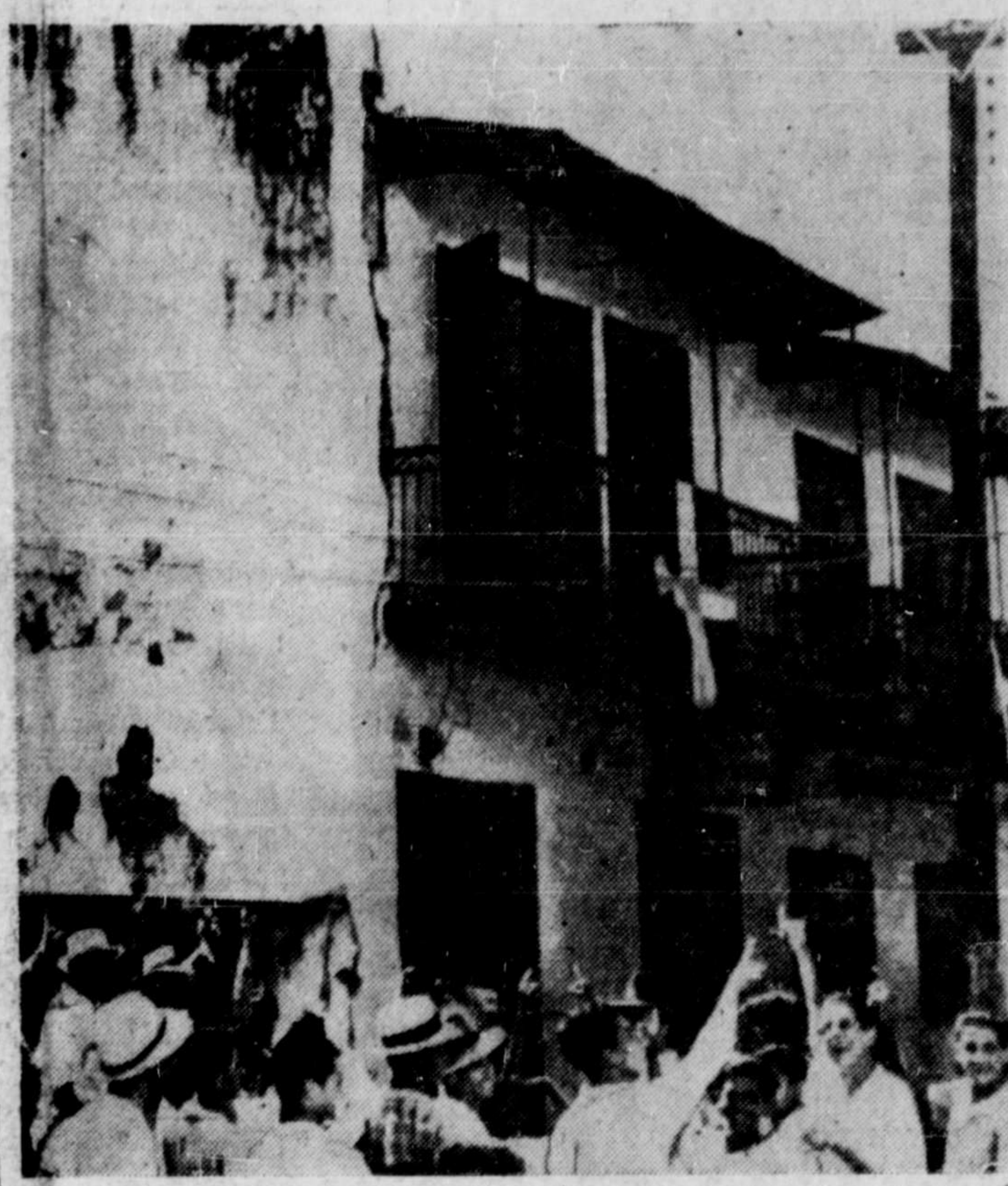
QUAKE IN DOMINICAN REPUBLIC—At the left side of the first balcony is a long crack in the wall of a building. Crowds at Ciudad Trujillo, Dominican republic, are pointing to its evidence of the long series of tremors which shook Puerto Rico and the Dominican republic. Despite the duration of the series of earthquakes a checkup has revealed comparatively small losses in the Caribbean area.
