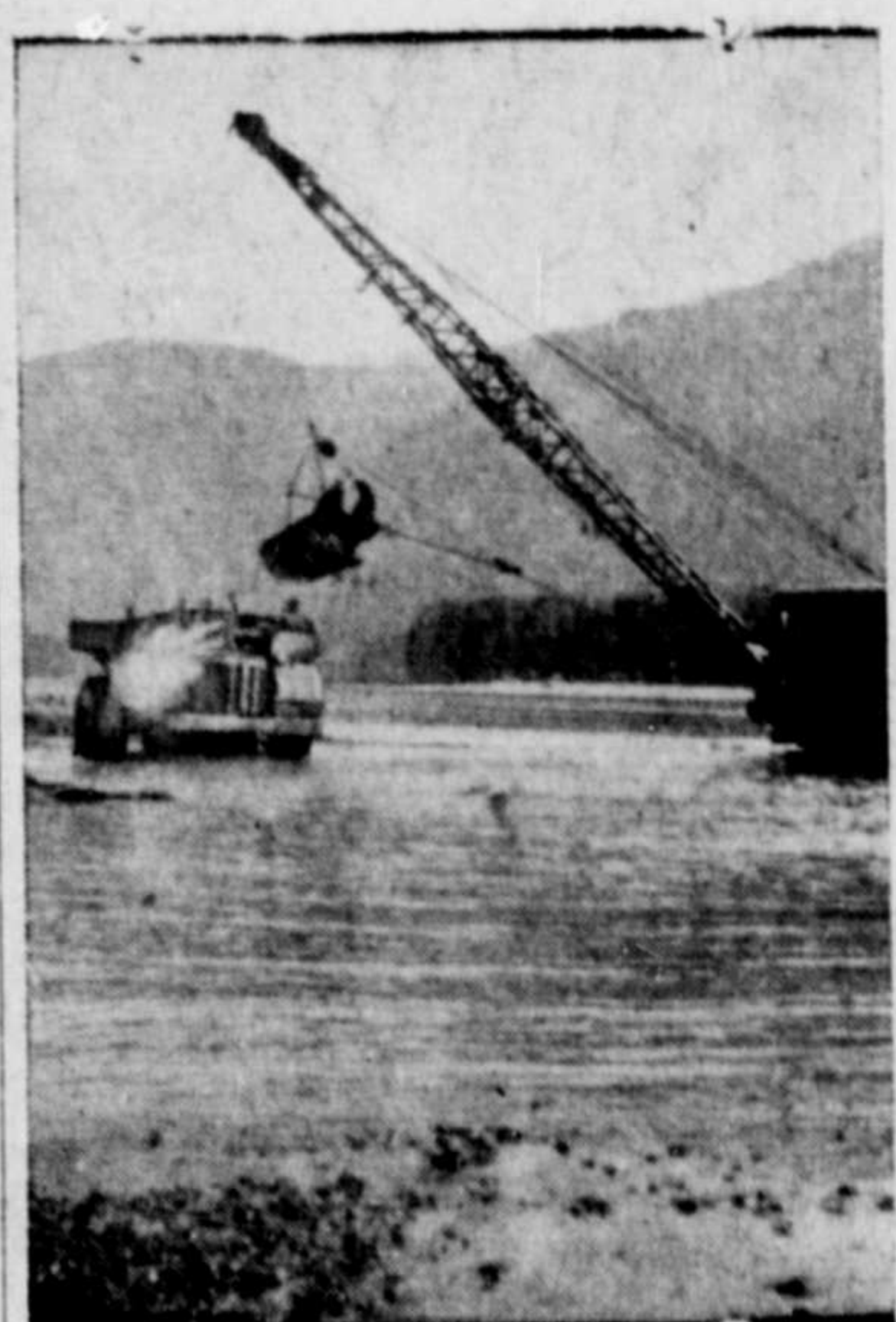
Dragline shovel loading a dumper with gravel for cushion from the Skeena River.
