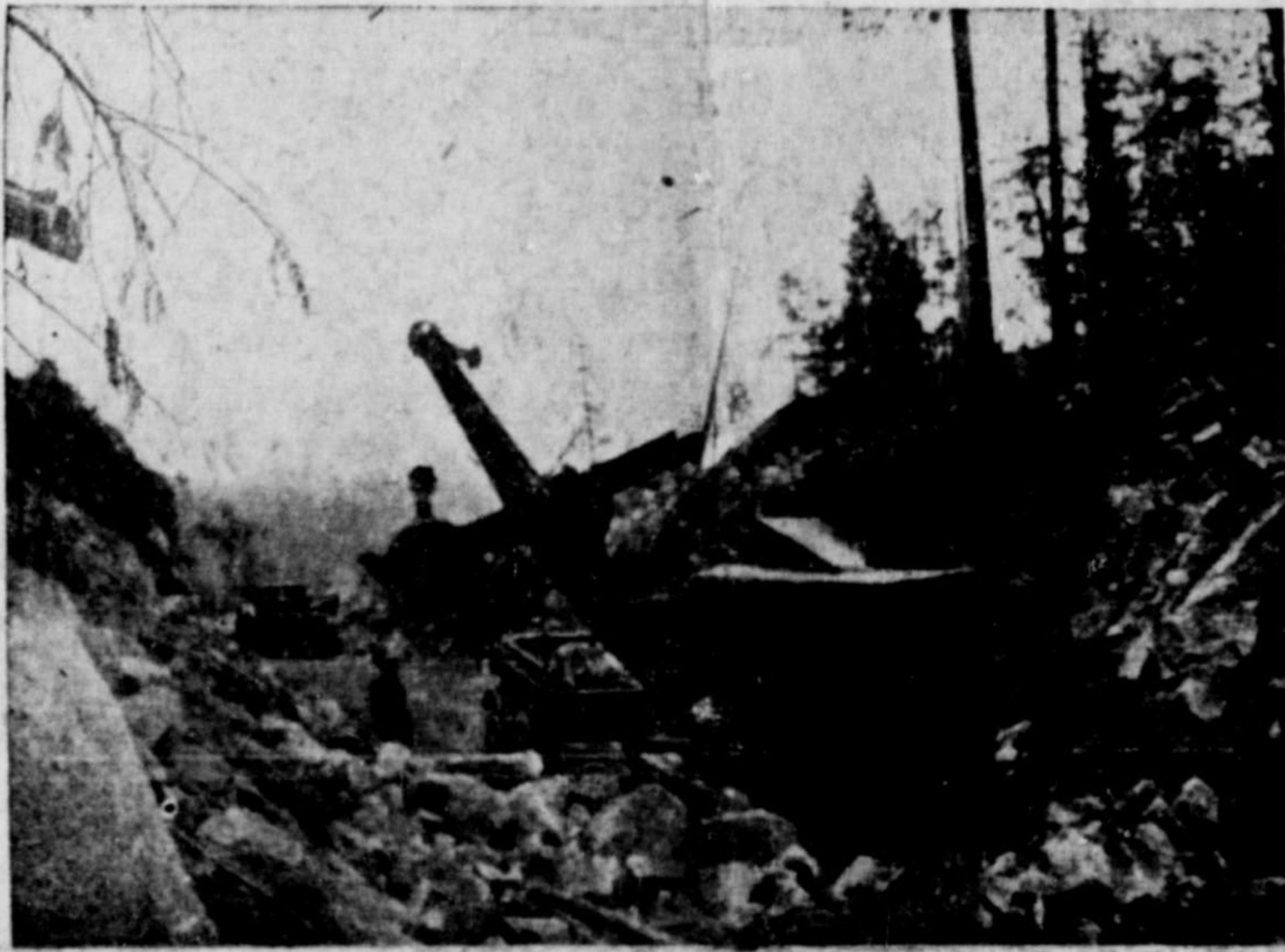
Power shovel dropping boulders into a dumper. The dumper was found a highly satisfactory carrying unit.
