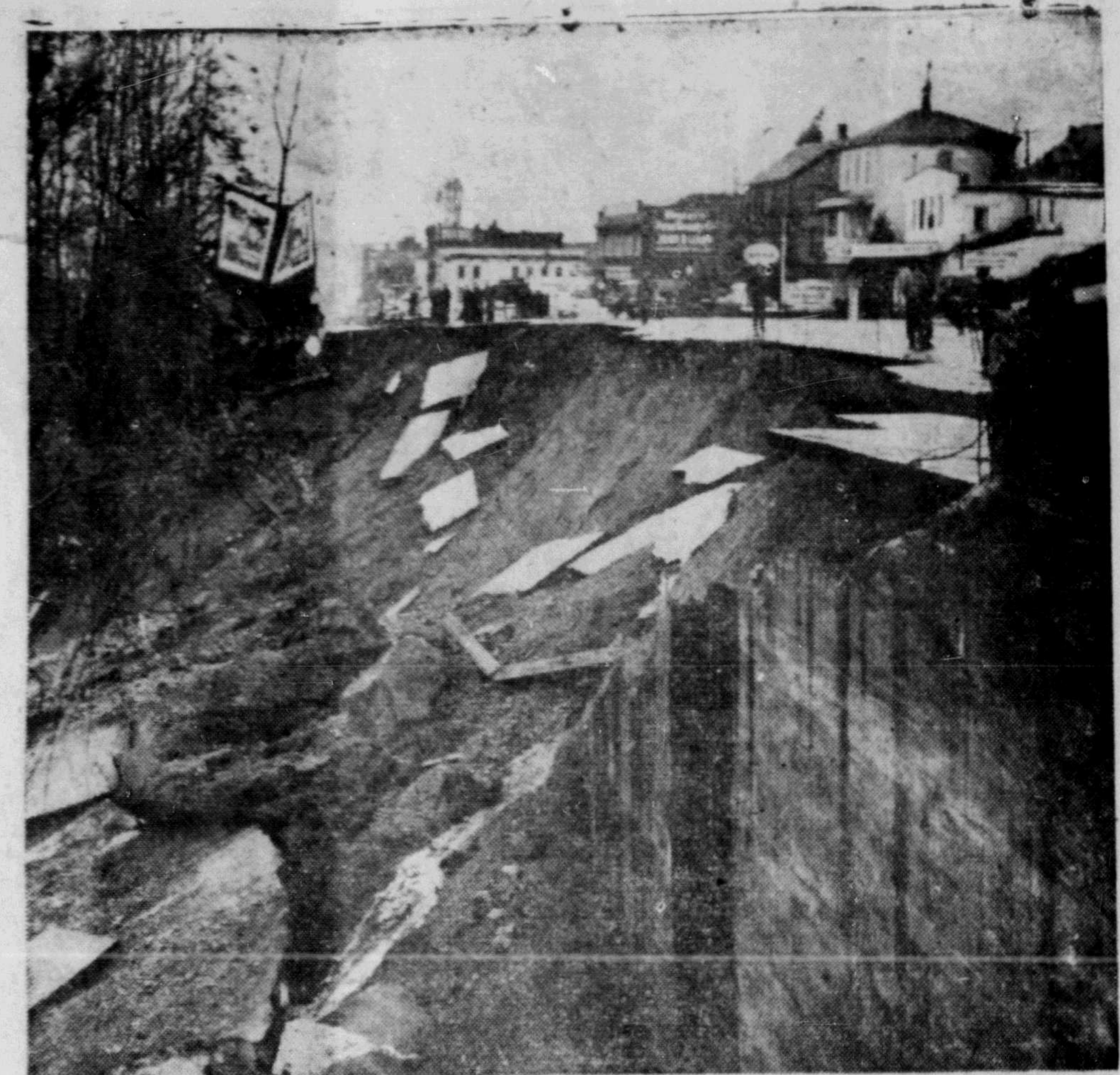
RETAINING WALL OUT —Heavy rains tore out more than 200 feet of retaining wall in New Westminster recently. Debris fell on the British Columbia Electric main line to the Fraser Valley and on Canadian National Railway spur line. The break was along Columbia, the city's main street. (C. P. Photo)
