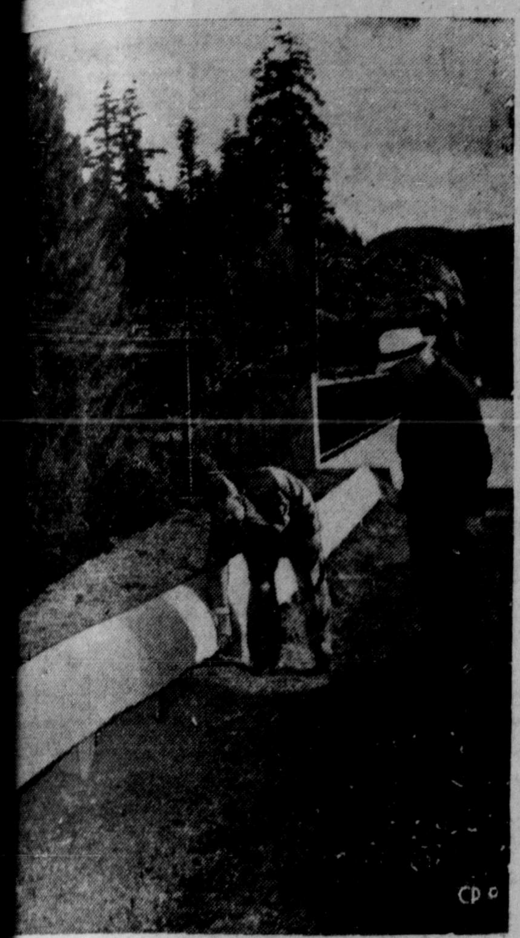
FOR SAFETY—British Columbia is the first province to install the new Danish-designed guard rail way safety. The concrete rail is curved so cars can't go through nor over. First installation is at the approach to the bridge on Vancouver Island's scenic Malahat Drive. District engineer, right, inspects the rail with W. S. [Name], the company which built it. (CP PHOTO)
