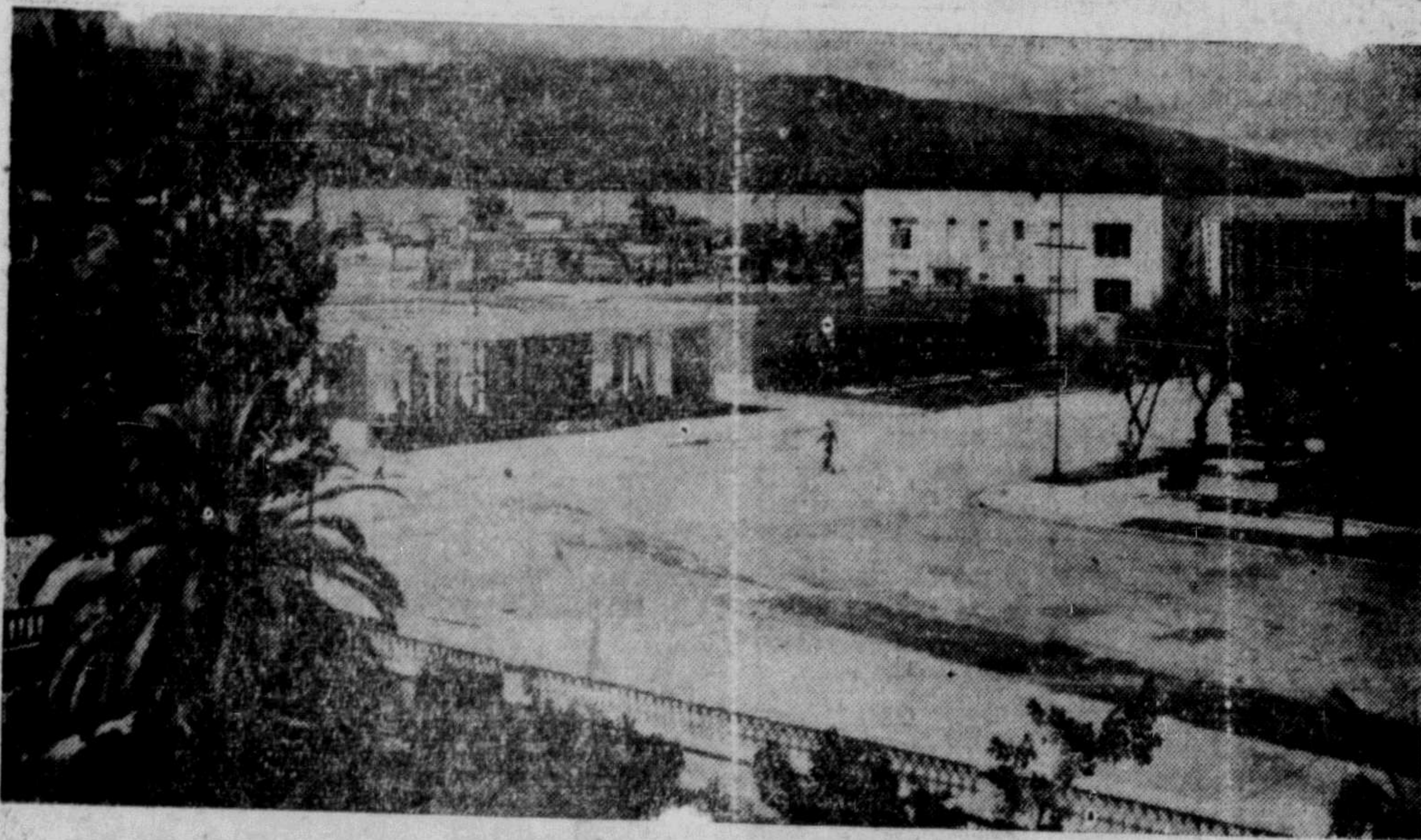
CARIBBEAN REPUBLIC TO STAGE WORD FAIR —A general view of the exposition grounds in Port au Prince, Haiti, showing progress of construction for the world's fair which is to open in December. The little Caribbean Republic, with only a 4,000,000 population is spending $25,000,000 on the fair which will have everything from industrial, agricultural and scientific exhibits to a gala entertainment area featuring, among other things, native voodoo dancing, cockfighting and performances by agricultural stars from the U. S. Many foreign governments are constructing booths on the exposition grounds.
