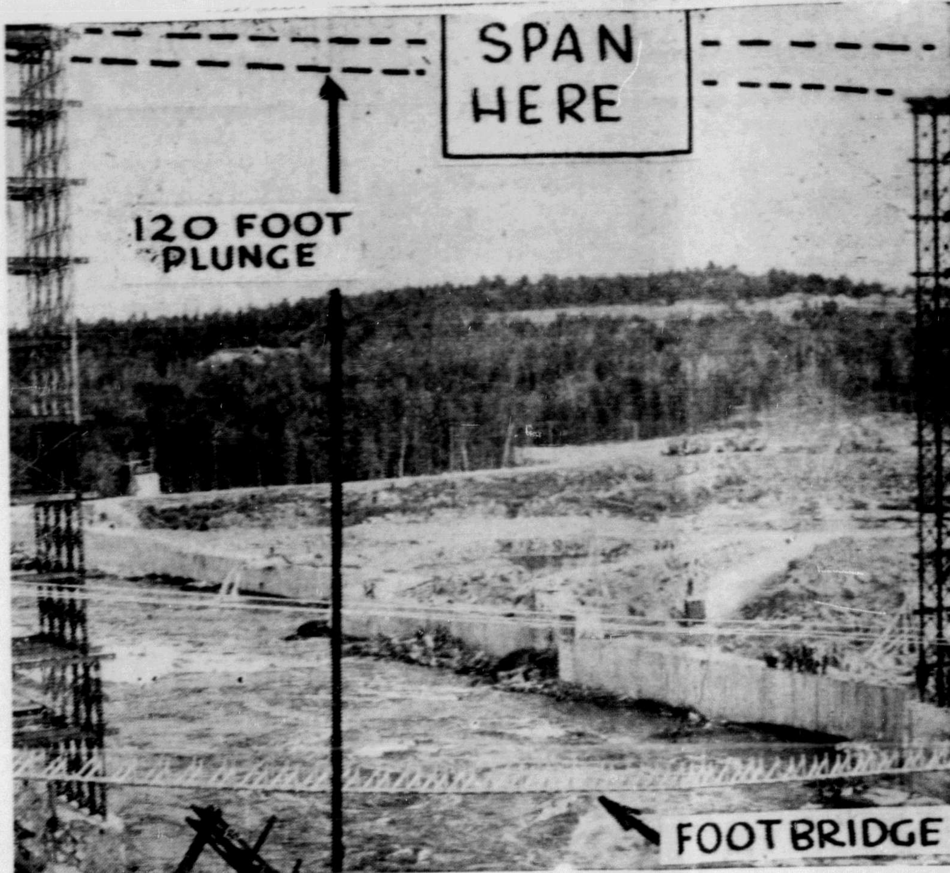
SIX MEN VANISH INTO OTTAWA RIVER AS DES JOACHIM'S BRIDGE COLLAPSES—Six Men plunged to their death in the Ottawa River when a 170-foot section of a Bailey bridge collapsed 20 minutes before quitting time. The tragedy occurred at the Ontario Hydro's $57,000,000 Des Joachim's power development project near Rolphton, Ont., approximately 150 miles north-east of Ottawa.
