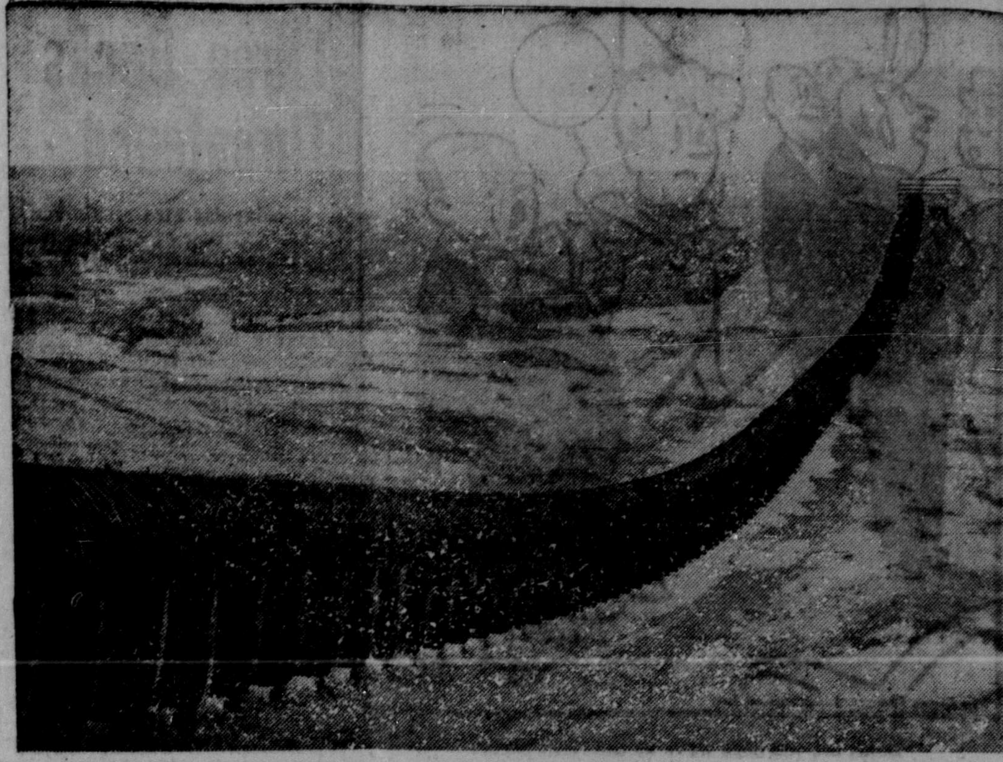
IRRIGATION PIPELINE — Rapidly nearing completion is this wood stave pipeline, built as a syphon across the Pinepound Coulee near the Alberta town of Spring Coulee for the main canal of the huge St. Mary-Milk rivers irrigation projects. A second syphon will be built later. With an inside diameter of 13 feet, it will carry 1,600 cubic feet of water per second across the coulee. Through its 960-foot length, the pipeline drops 60 feet and then rises that height again. (CP Photo)
