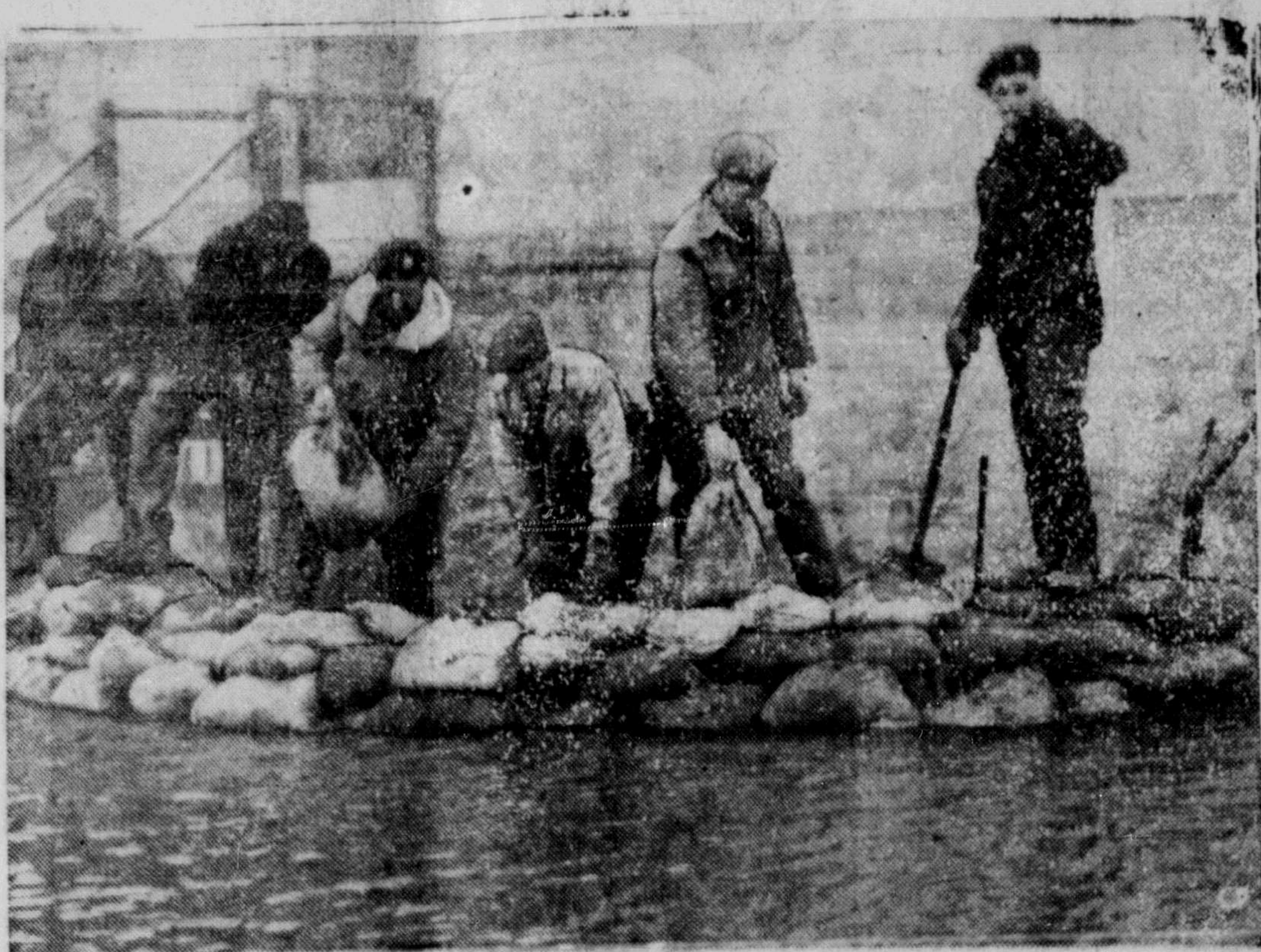
SANDBAGGING HOSPITAL—Soldiers of the Winnipeg area took over dyking operations when civilian workmen became exhausted, and kept flood waters from forcing seriously-ill patients and expectant mothers from the hospital at Morris, Man. By Monday morning, the soldiers had strengthened the dyke and increased its height above the level of the flood waters. (CP Photo)
