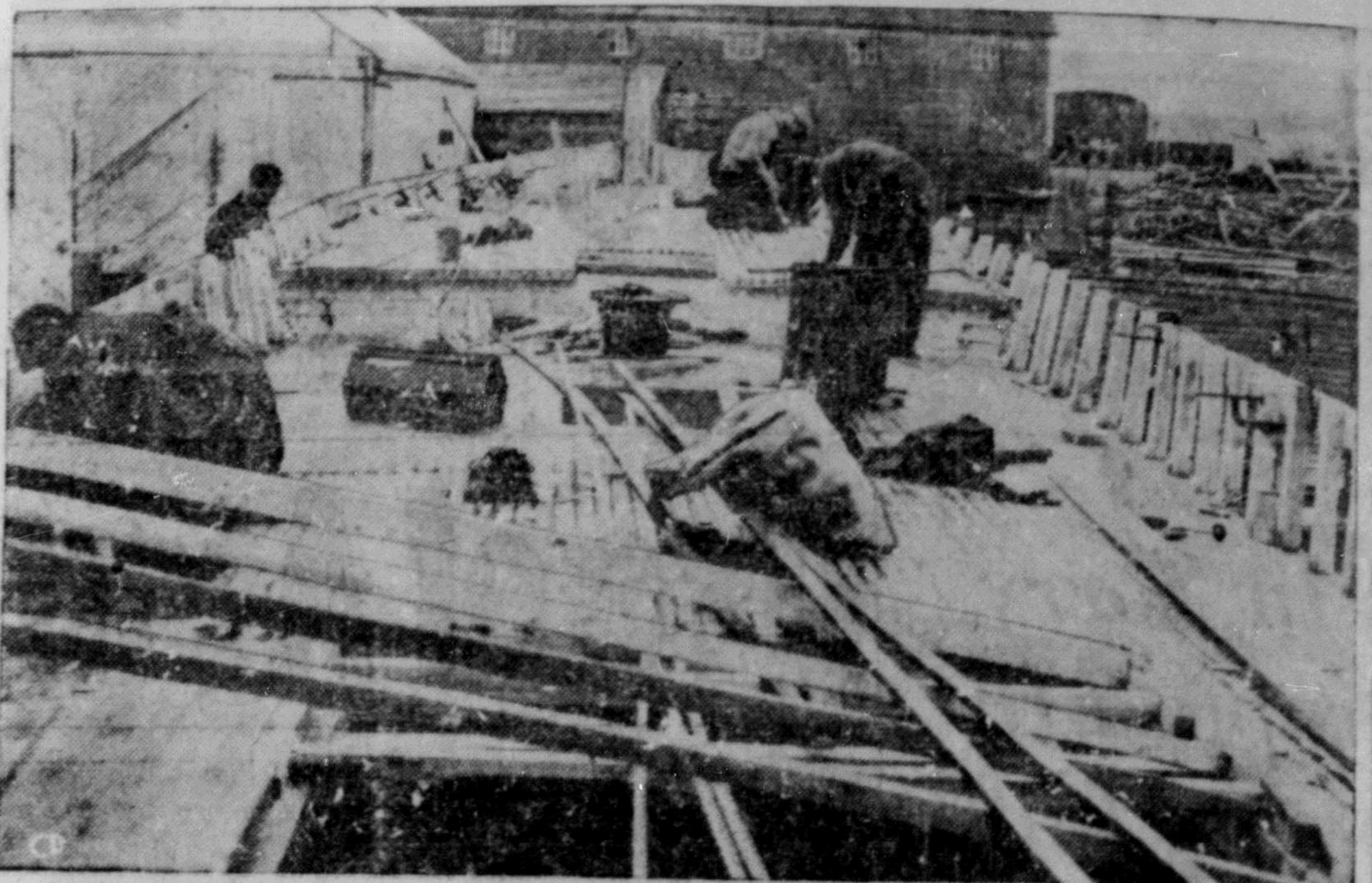
"LUKIE'S BOAT"—Shipbuilders in the yards at Clarenville, Nfld., work on a new-type fishing boat. Construction of the vessel is part of a drive for modernization of the province's fishing industry. Unofficially called "Lukie's Boat"—the name of an island folk song—she is modelled on the Norwegian-type fishing boats and is intended for use in comparatively rough waters. (CP PHOTO)
