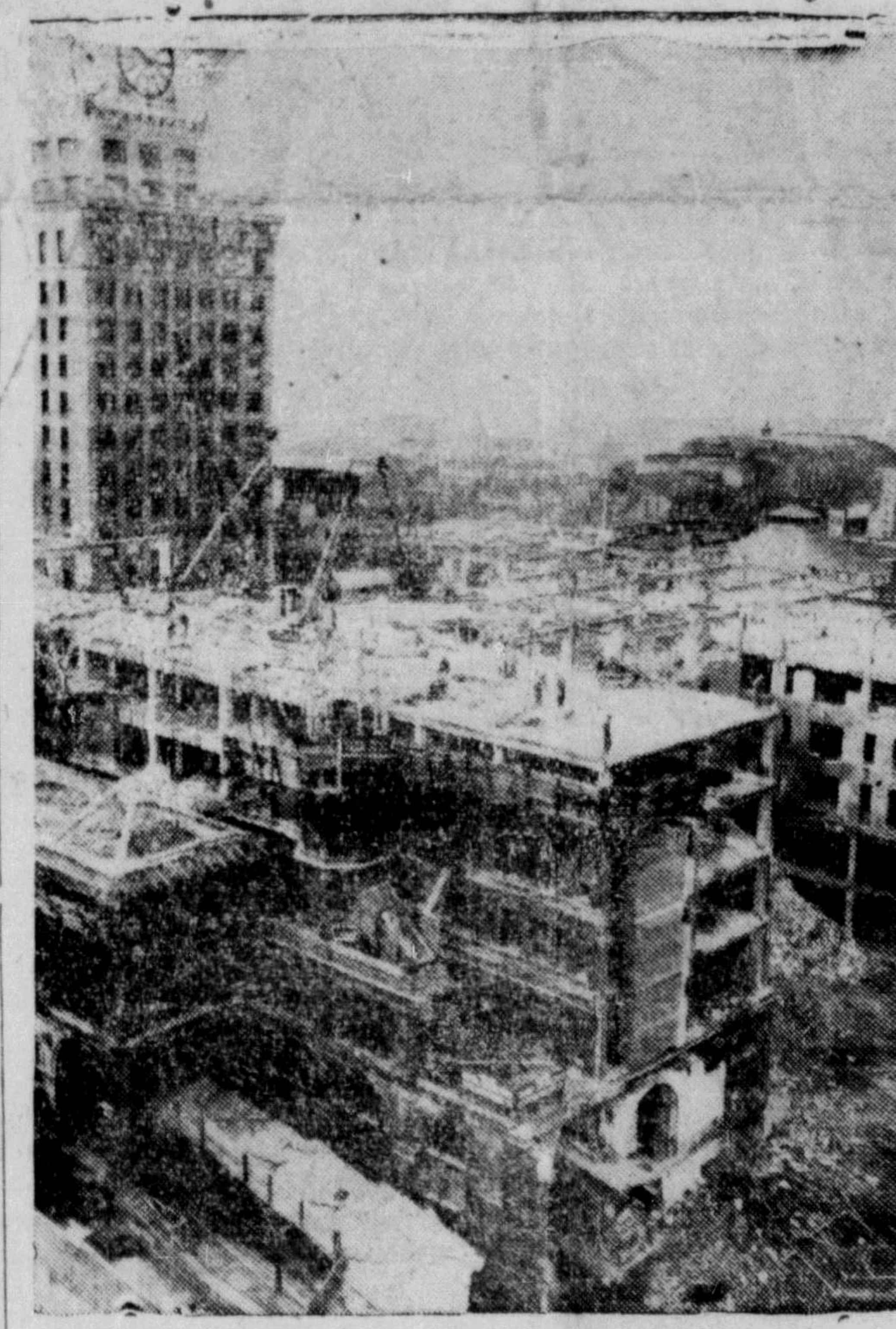
VANISHING LANDMARK—Vancouver's skyline won't look the same when wreckers complete the job of razing the old Vancouver Hotel, long a city landmark. It is expected that demolition of the huge building, begun three months ago, will be finished by mid-October. (C. P. Photo)
