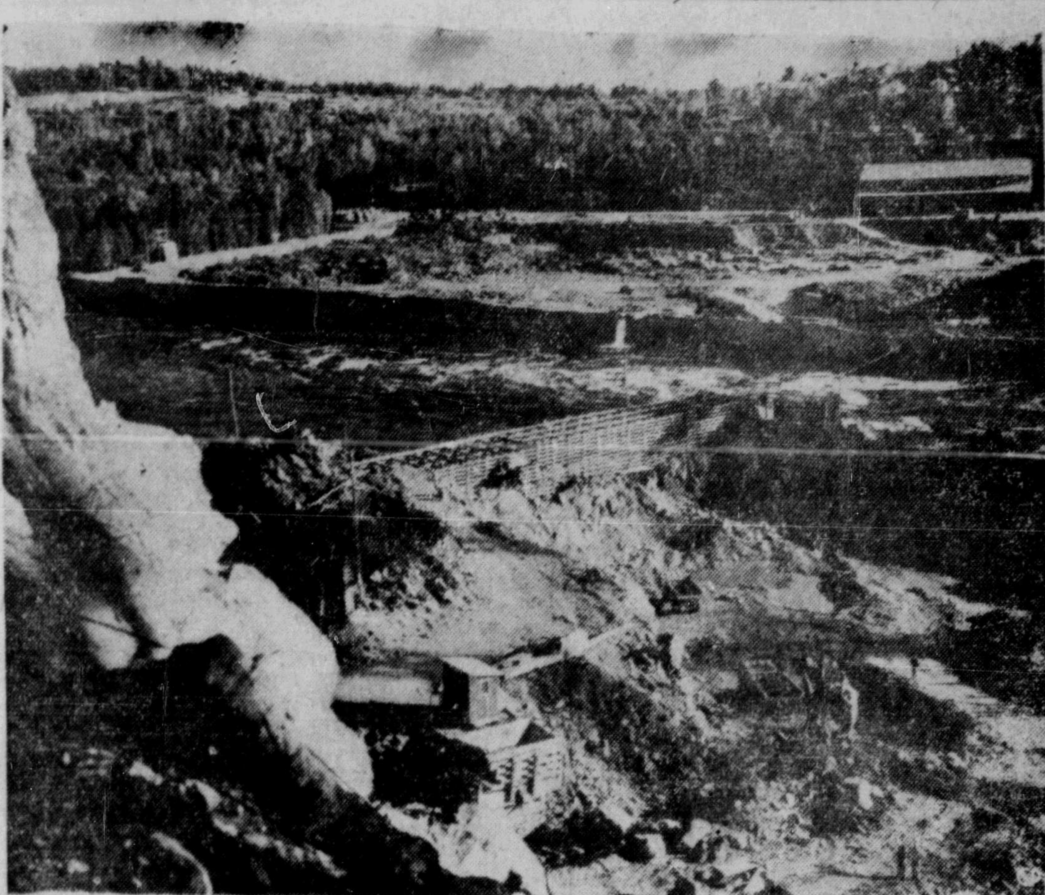
BIG POWER PROJECT—One of the largest power projects now under construction in eastern Canada is the Des Joachims development on the Ottawa River, 140 miles from the capital. Work is proceeding during the winter. This Department of Mines and Resources photo shows one of the diversified operations necessary to build the dam. (CP Photo)
