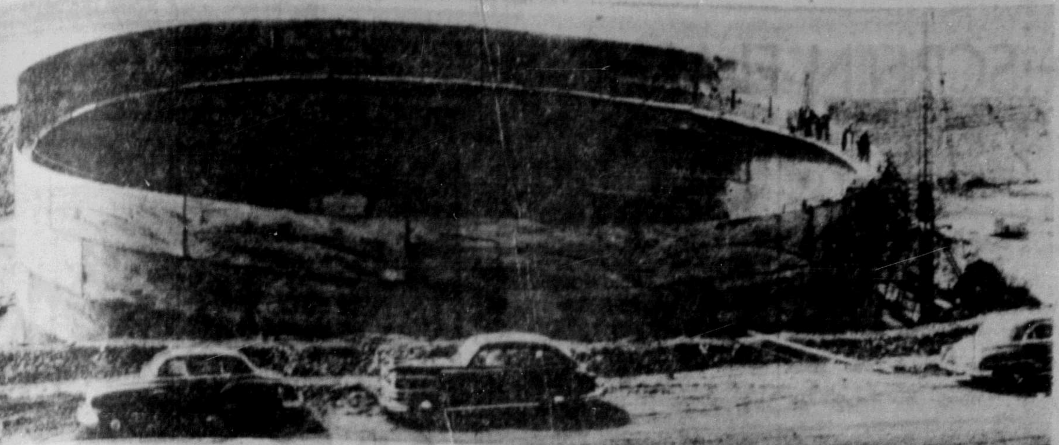
PROGRESSING ON SCHEDULE at Trans Mountain Line Company crude oil tank farm at Burnaby. This shows construction of the first 150,000-barrel tank. The steel plate sections are 8 feet by 30 feet. As quickly as they are raised in place, they are welded from the outside and inside. There are six "rings" to each of the 48-foot tanks.
